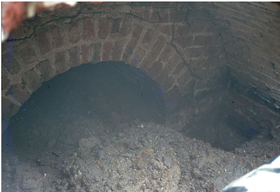
Figure 5. Culvert F58 entering the east end of the main south moat culvert.
