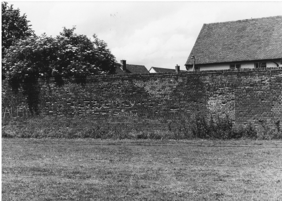
Figure 22. The north wall of the eastern end of the central garden in 1986 showing the blocked door.
