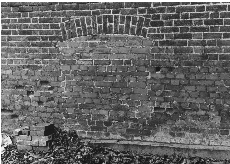
Figure 67. The blocked door at the north end of the east boundary wall of the present south garden. East side of the wall.
