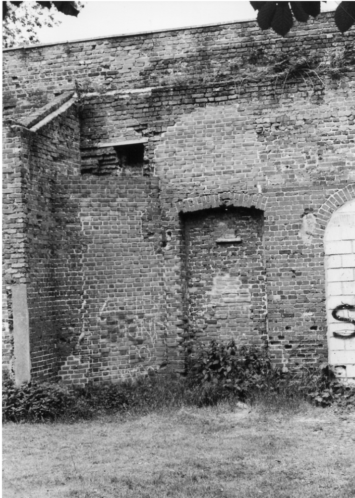
Figure 49. The fireplace and flue in the north-west corner of the building at the east end of the wall.
