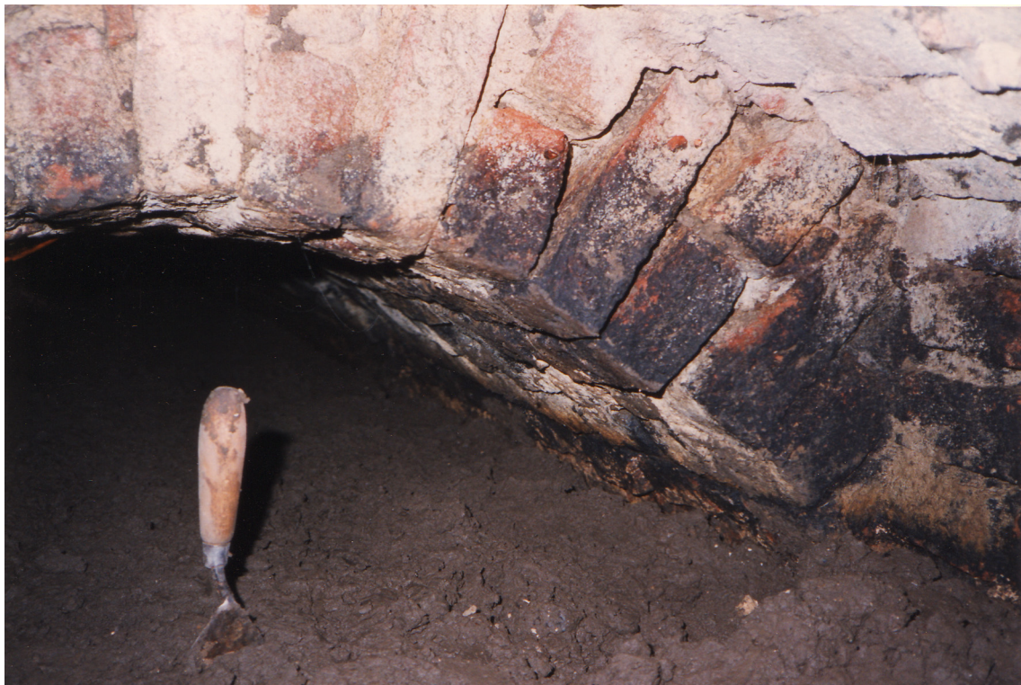
Figure 4. The drop in the roof of culvert F58. (Photo Roger Browne.)
