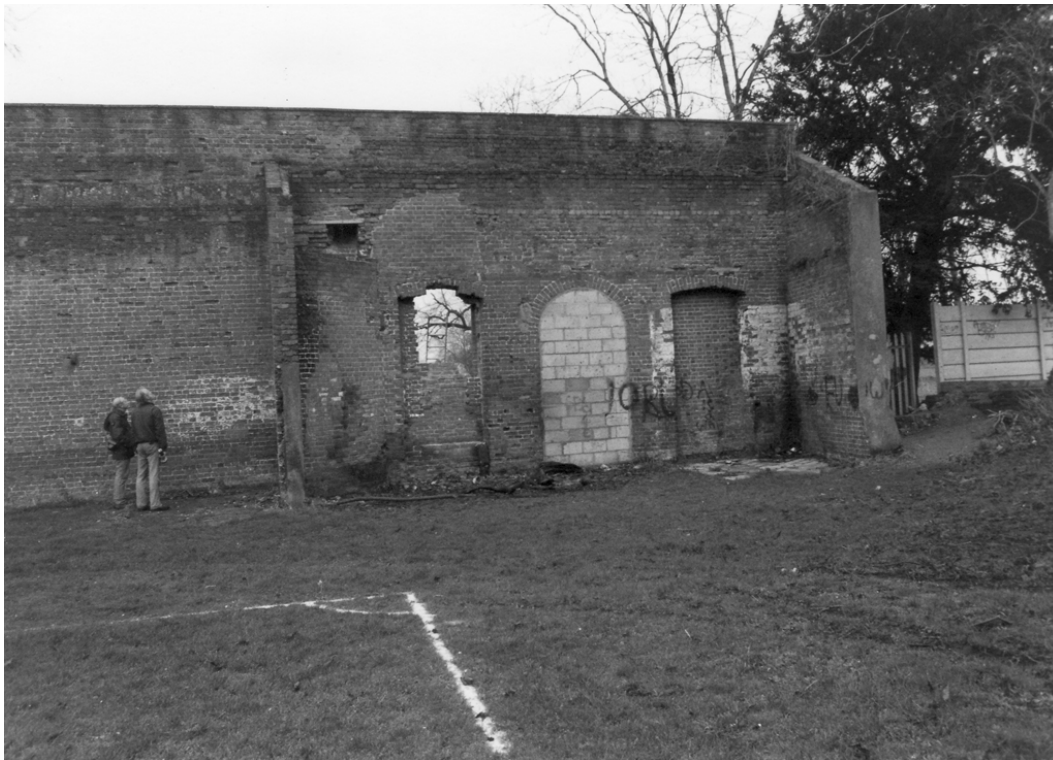
Figure 45. The south side of the east end of the wall on 10 January 1988. The blocking of the western window has been demolished.
