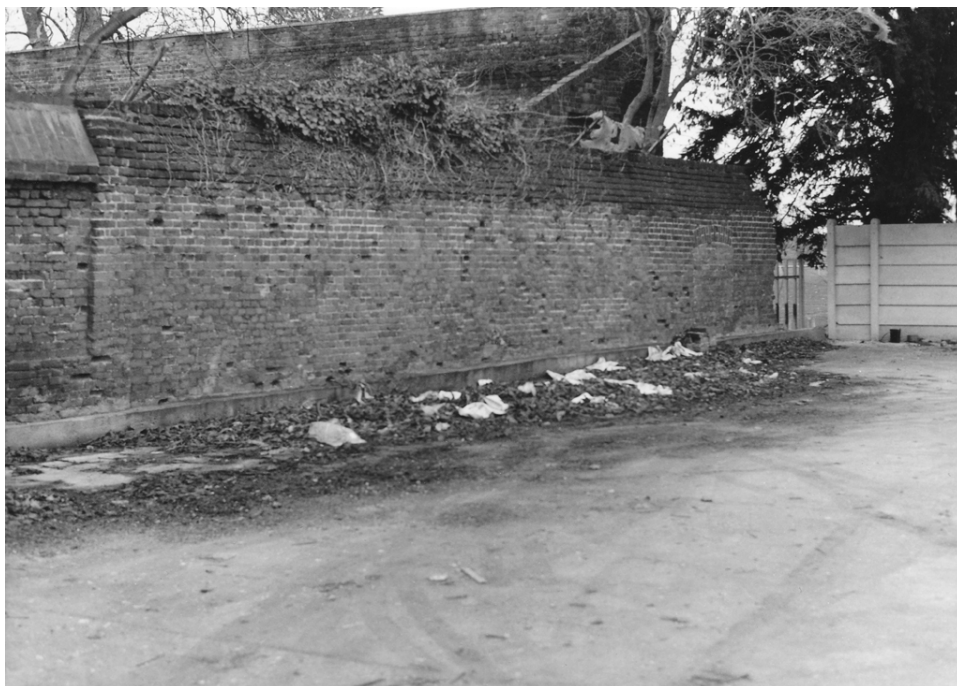
Figure 66. The north end of the east boundary wall of the present south garden with the Orangery wall in the background. Note the blocked door at the north end of the wall.
