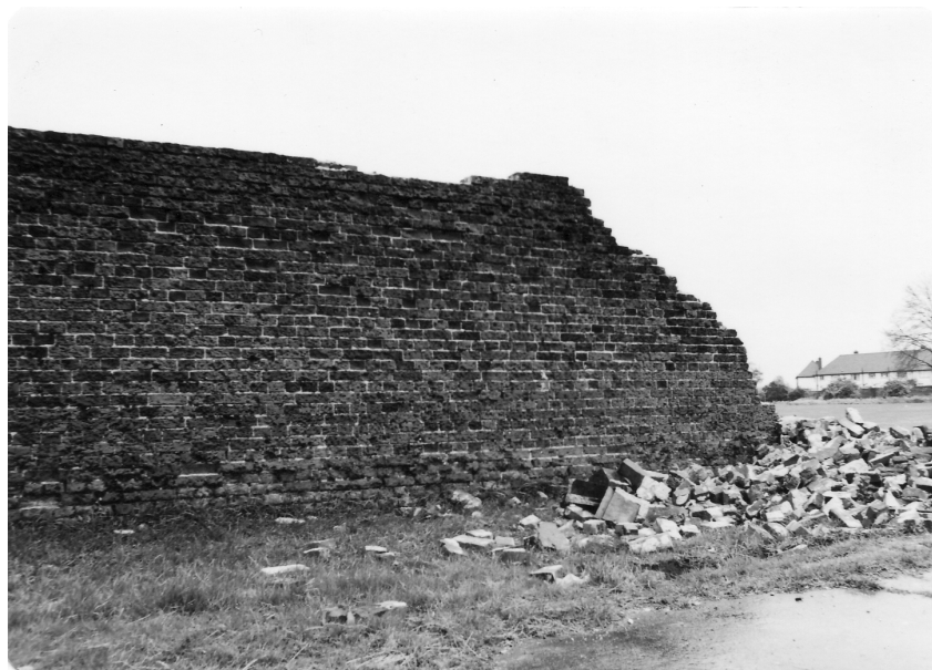
Figure 19. The remains of the wall between the north gate and river on 3 May 1981. Note the bond break adjacent to the gate pier.
