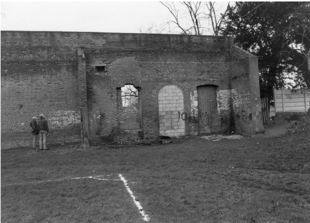
Figure 14. The south side of the east end of the wall on 10 January 1988. The blocking of the western window has been partly demolished.
