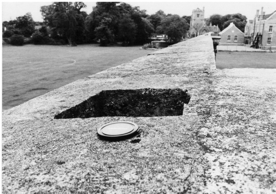
Figure 19. Looking west along the top of the orangery wall from the second pilaster, 1985. The flue in the foreground rises from the fireplace shown above.
