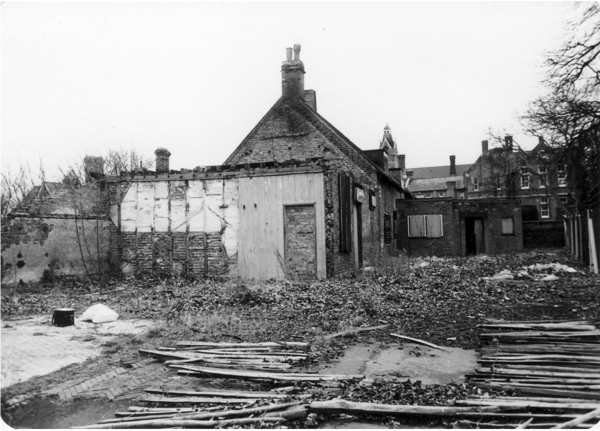
Figure 88. Looking south across the site of 2A to the lower part of 2B. The modern extension to the west side of the changing rooms can be seen background right. Yellow filter. 1 March 1981.
