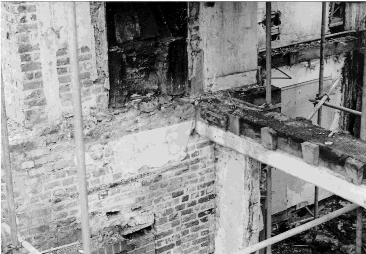
Figure 40. The north side of the eastern chimney-stack around first floor level showing the bridging joist which supported the floor of rooms 1-10 and 1-11. The fireplace heated room 1-11. Part of the fireplace of room 1-5 is visible at the bottom of the photo. During conversion work.
