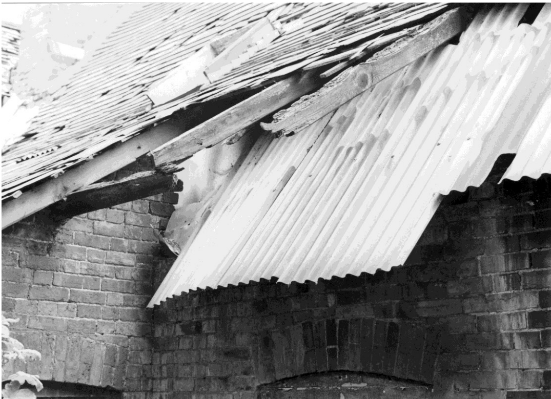
Figure 36 The east wall of room 1-4 with exterior wall or room 1-5 on the left. 1983. The corrugated iron appeared to have been inserted as a bodge repair to protect the head of the wall following the decay of the roof of the extension against the wall of room 1-4.
