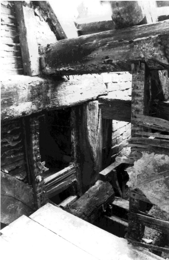
Figure 73. Head of post 2E with the tie-beam of truss 2 to the left. The beam added to support the roof extension of room 1-5 can be seen at the top. The floor room 1-10 at the bottom. Looking northeast. March 1983.
