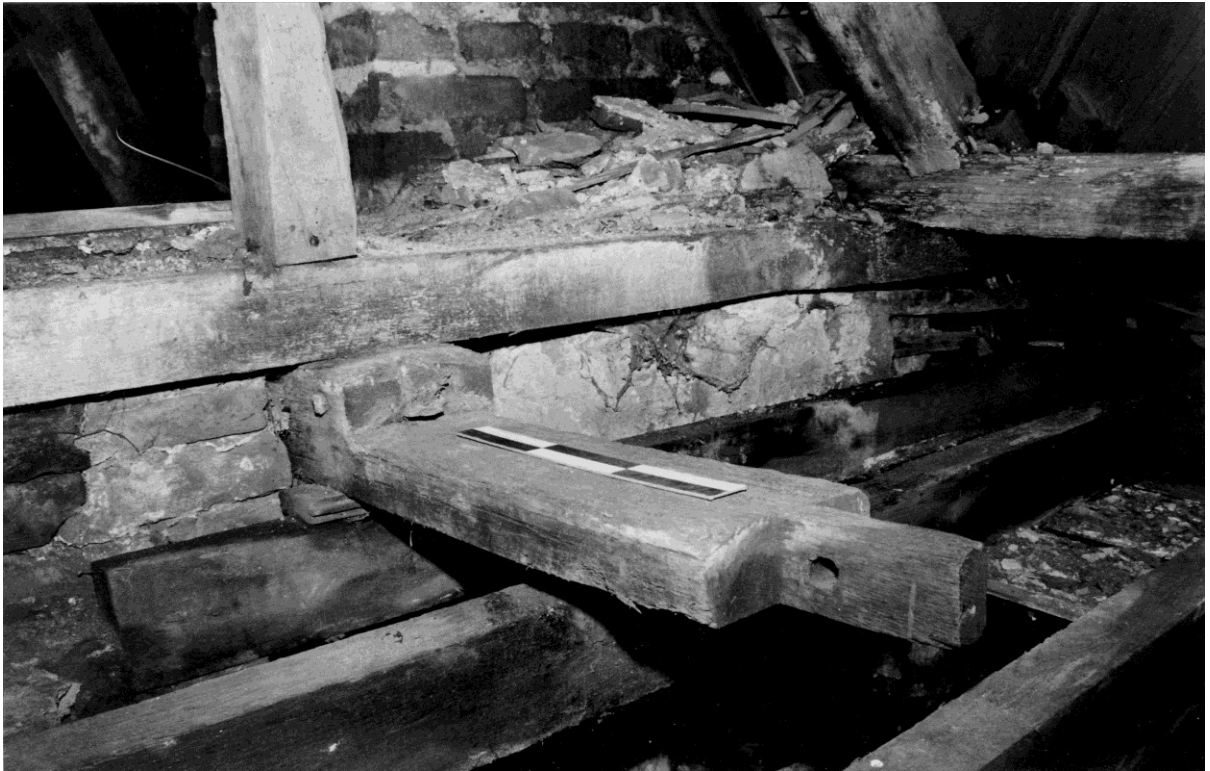
Figure 5. The scarf at the south end of the surviving length of collar purlin looking roughly northeast. The joint was located above room 1A-7 close to the north wall of the room. Scale in 30cm long.
