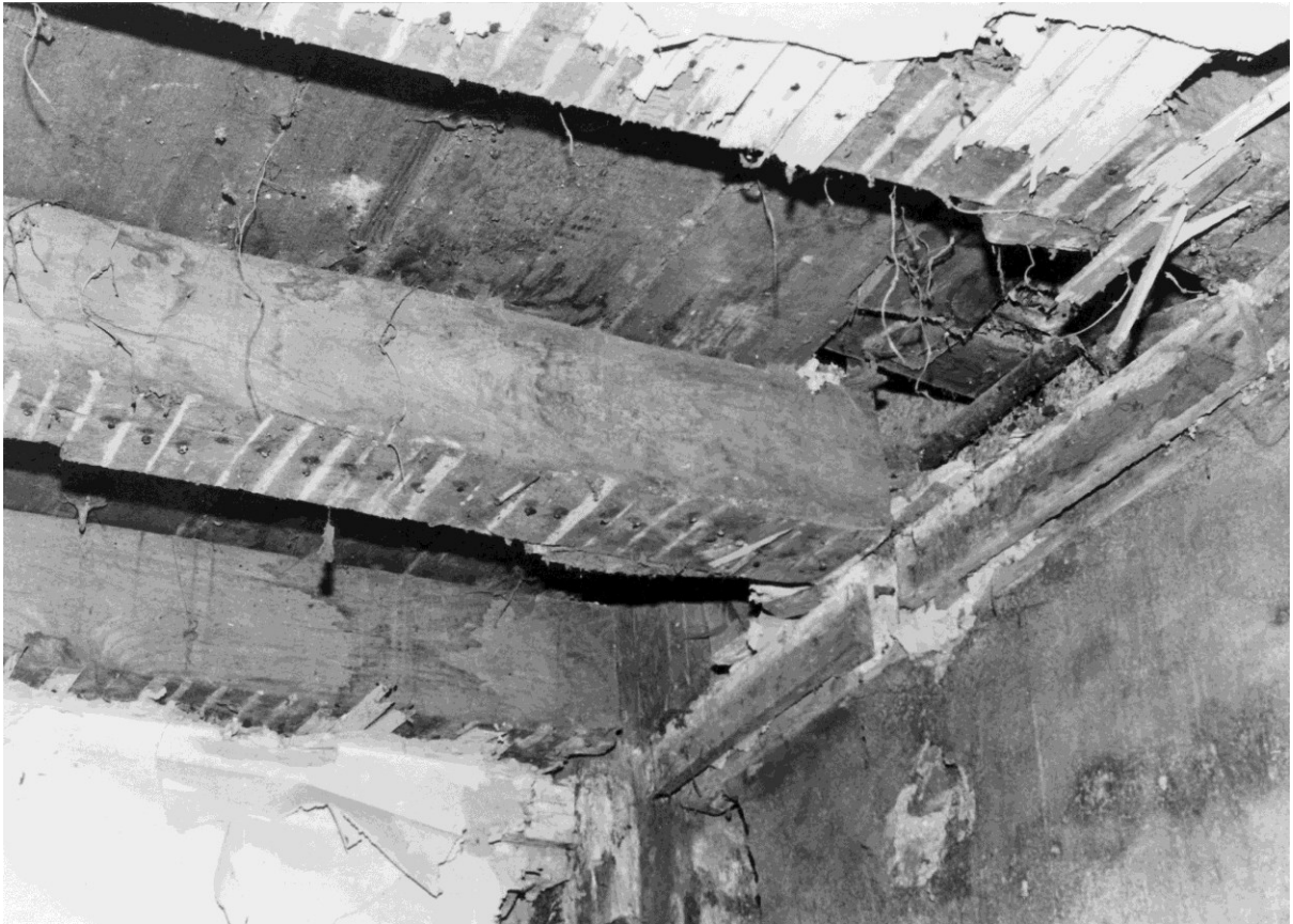
Figure 74. The ceiling at the southwest corner of room 1-6 showing the bodged repairs to fill the gap between the joists and the west wall.
