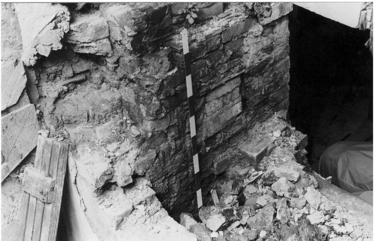
Figure 57. The east side of the east chimney-stack by the ovens. Note the blocked flue to the right of the scale.
