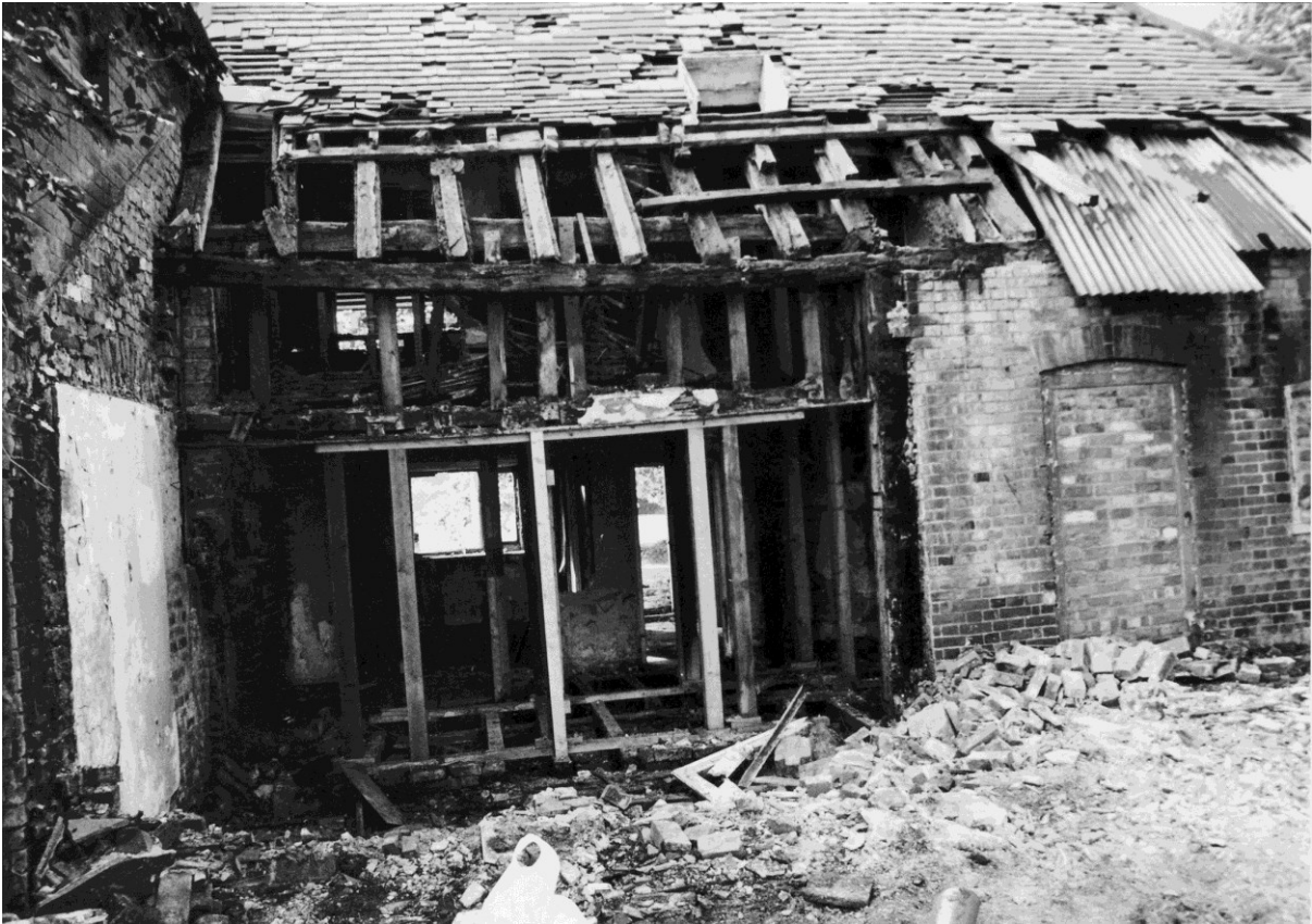
Figure 37. The exposed timber frame of the east wall of room 1-5 during conversion in 1986.
