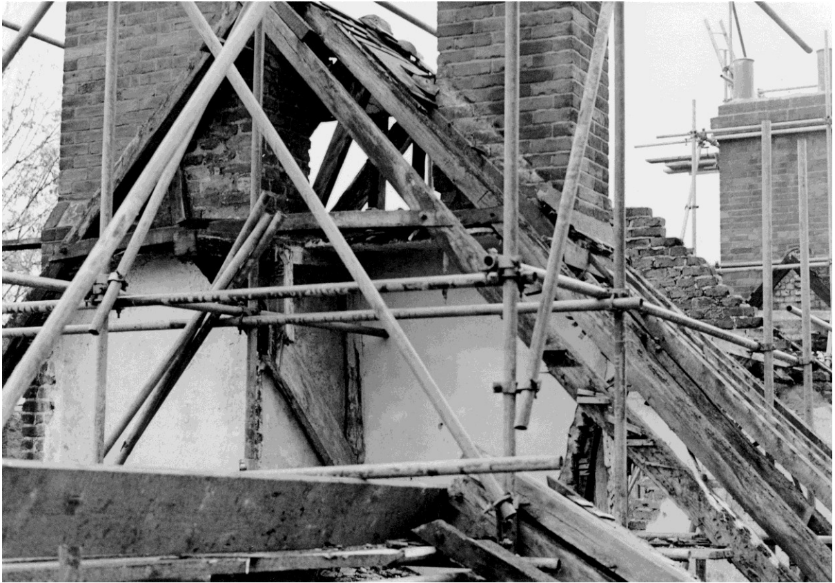
Figure 4. The sawn-through collar purlin and the brace to crown post 2 seen during conversion work in 1986-7. Looking approximately south.
