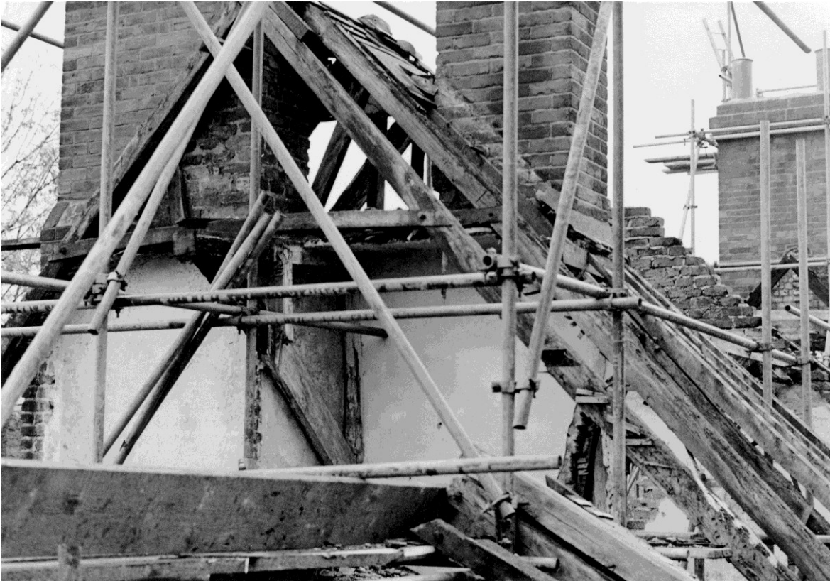
Figure 39. The east and west chimney-stacks showing the relationship to the roof during conversion work.
