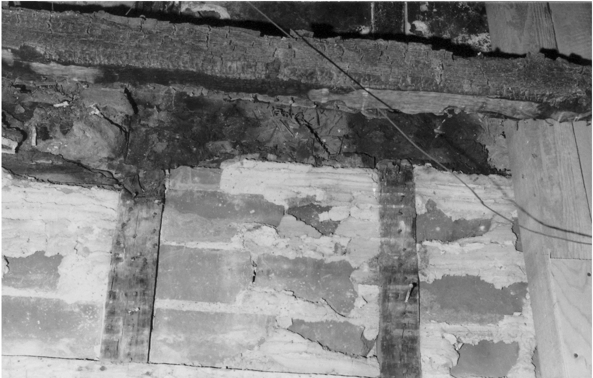
Figure 75. The upper part of the north wall of room 1-1 showing the boundary between the wattle and daub above and the timber framed brick work below. The timber across the top was one of the floor joists for room 1-11. The wattle and daub continued upwards to form the north wall of 1-11 which was part of truss 2.
