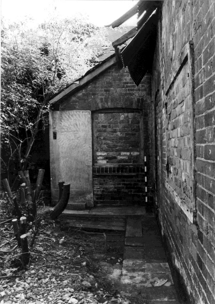
Figure 33. The east side of the cottages looking south from the northeast corner towards the extension of room 1-5. The foundations of the structure built against the east wall of room 1-4 are in the foreground.
