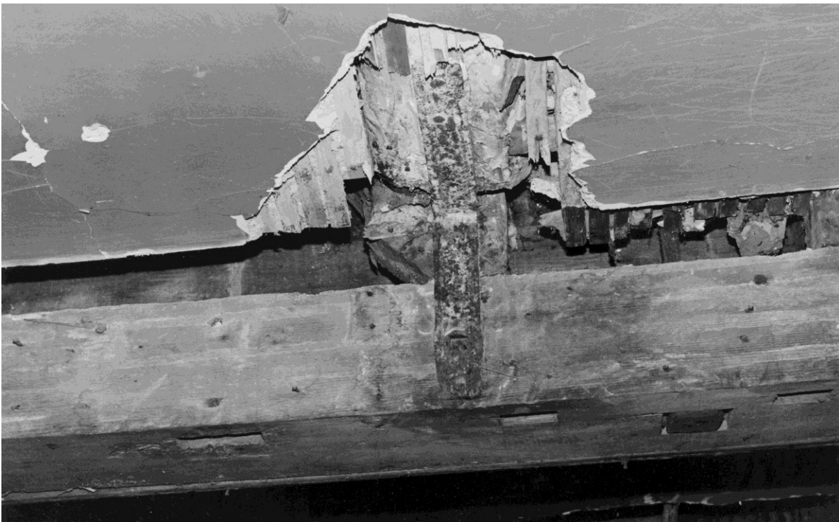
Figure 69. The ceiling of room 1-4 looking east showing the bridging joist which runs below the wall dividing rooms 1-8 and 1-9 (running right to left across the photo) and the metal bracket which supports the subsidiary east-west running bridging joist for the floor of 1-8.
