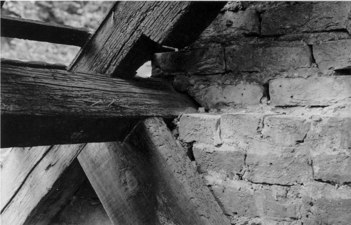
Figure 84. The west side of the north truss of 1B showing junction of queen post with principle rafter. 29 August 1982.
