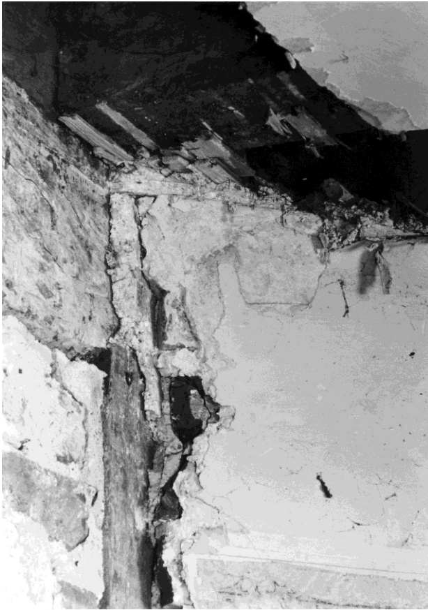
Figure 44. The southeast corner of room 1-6 at ceiling level. The plastered area to the right is the edge of the fireplace which was built into the corner of the room. The timber to the left is the bridging joist which supported the first floor in bay 2. The brickwork under it is the wall between rooms 1-6 and 1-5. Note the plaster on the side of the bridging joist showing that it and the wall were earlier than the fireplace.
