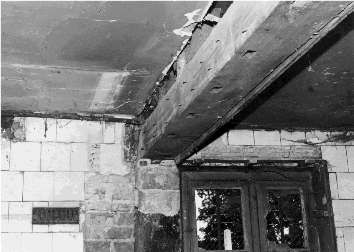
Figure 68. Ceiling of room 1-4 looking north showing the bridging joist below the wall between 1-8 and 1-9. Post 1C can be seen below the joist by the window. 1983.
