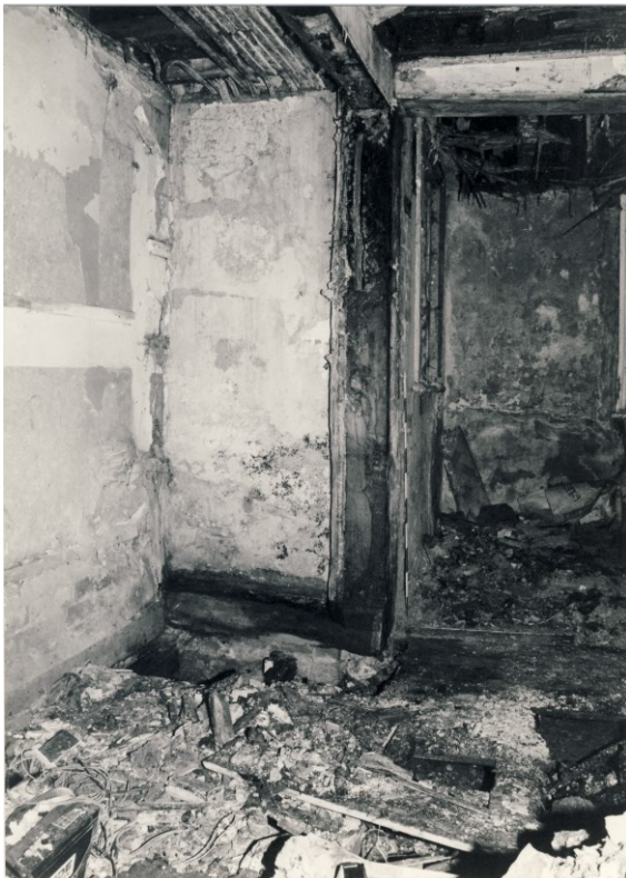
Figure 19 (above). The west side of post 2E with the surviving section of ground sill.
