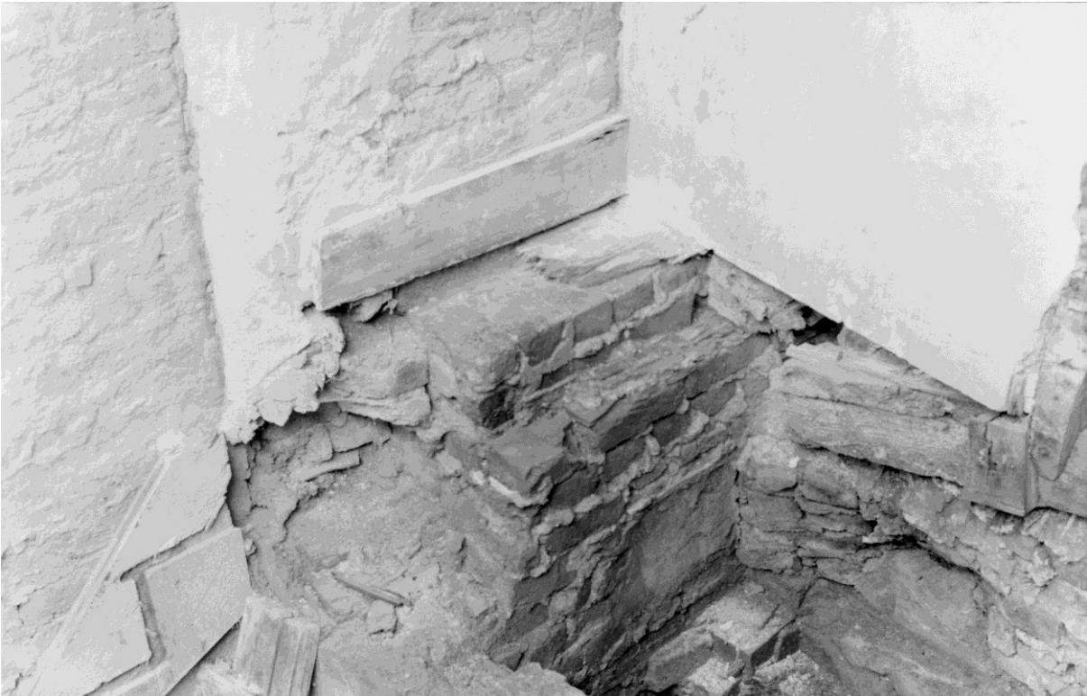
Figure 46. The north side of the chimney-stack above the oven. Note the lath, plaster and tile packing on the lower ledge which originally supported the first floor. The skirting and floorboard on the upper ledge appear to relate to a staircase which was constructed over the oven probably after it had gone out of use.
