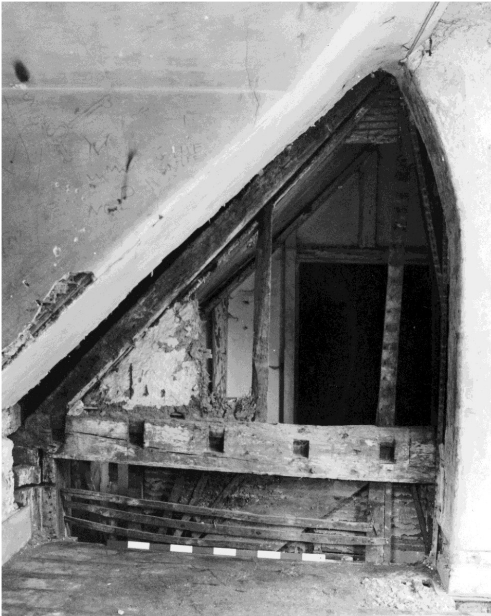
Figure 80. The west end of the south side of truss 3 in room 1A-7. Note the lath and daub and the mortises for floor joists at attic level.
