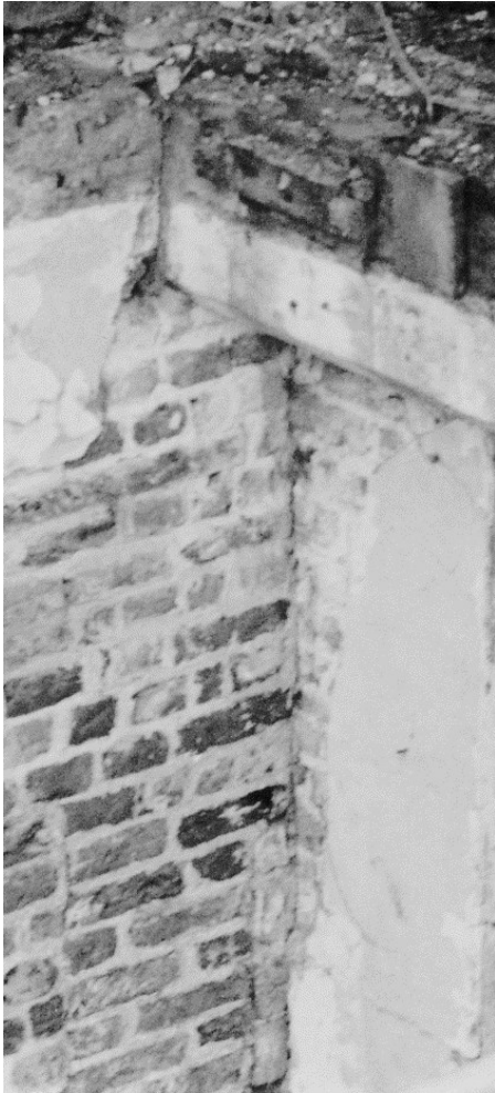
Figure 41. Detail of figure 40 above showing the butt joint between the chimney-stack (left) and the bridging joist and the wall beneath it.
