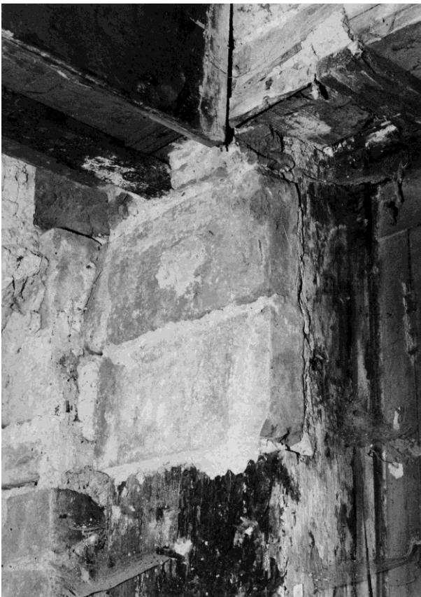
Figure 59 (left). The south side of post 1C below the first floor. Note the brick filled notch cut into the timber probably to hold a bridging joist below the level of the existing floor.
