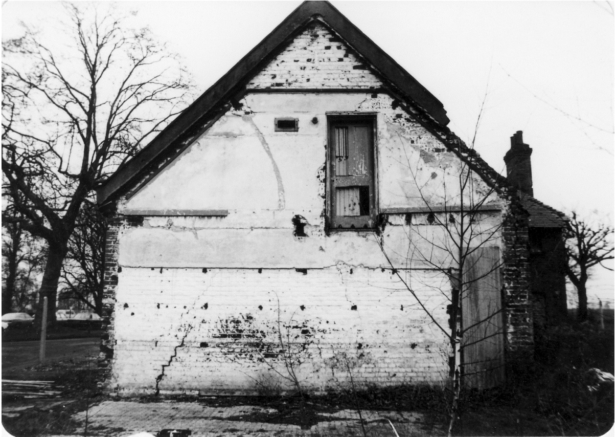
Figure 85. The south end wall of number 2 looking north on 1 March 1981 before the fire.
