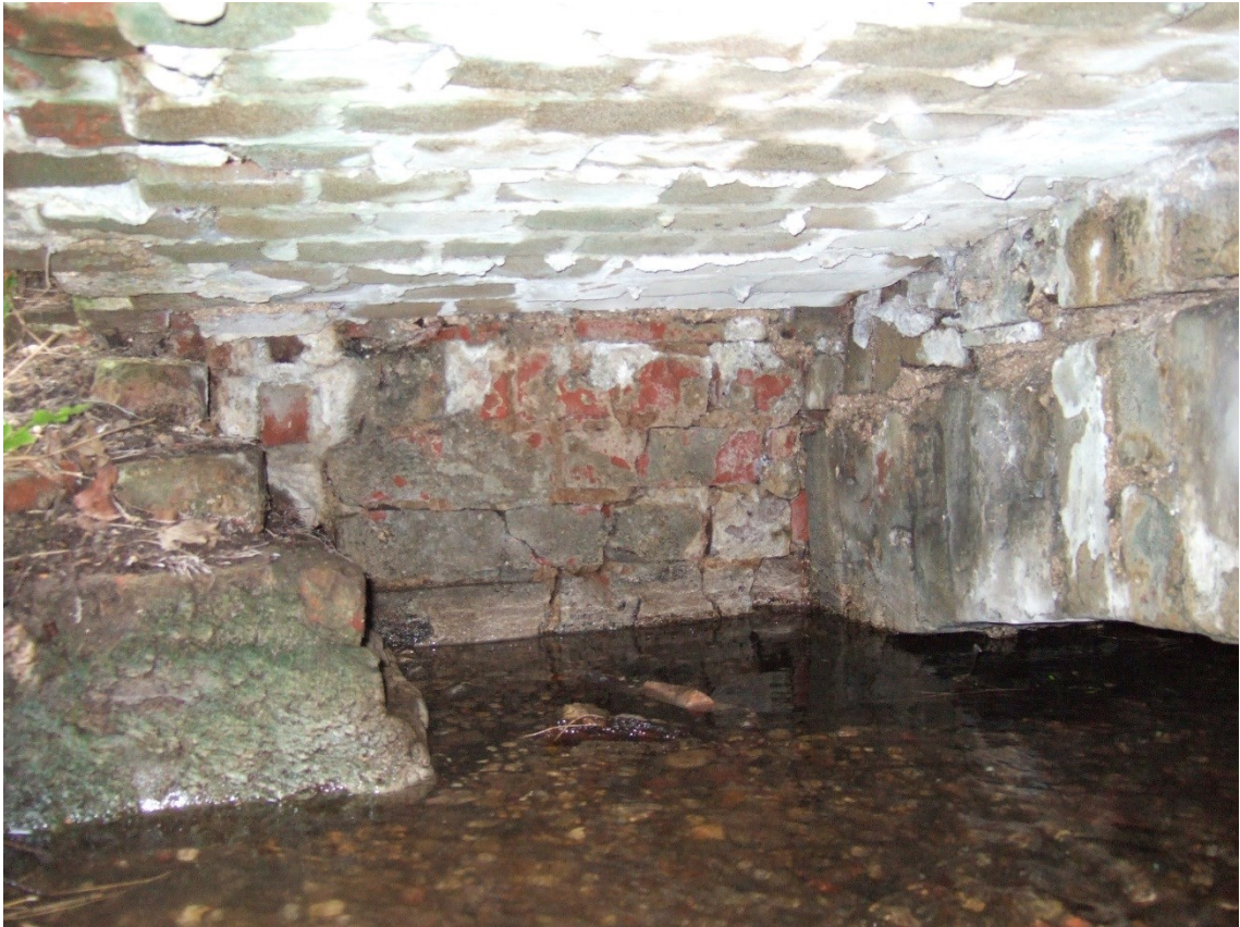
Figure 10. The north side of the entrance to the culvert under the lawn.
