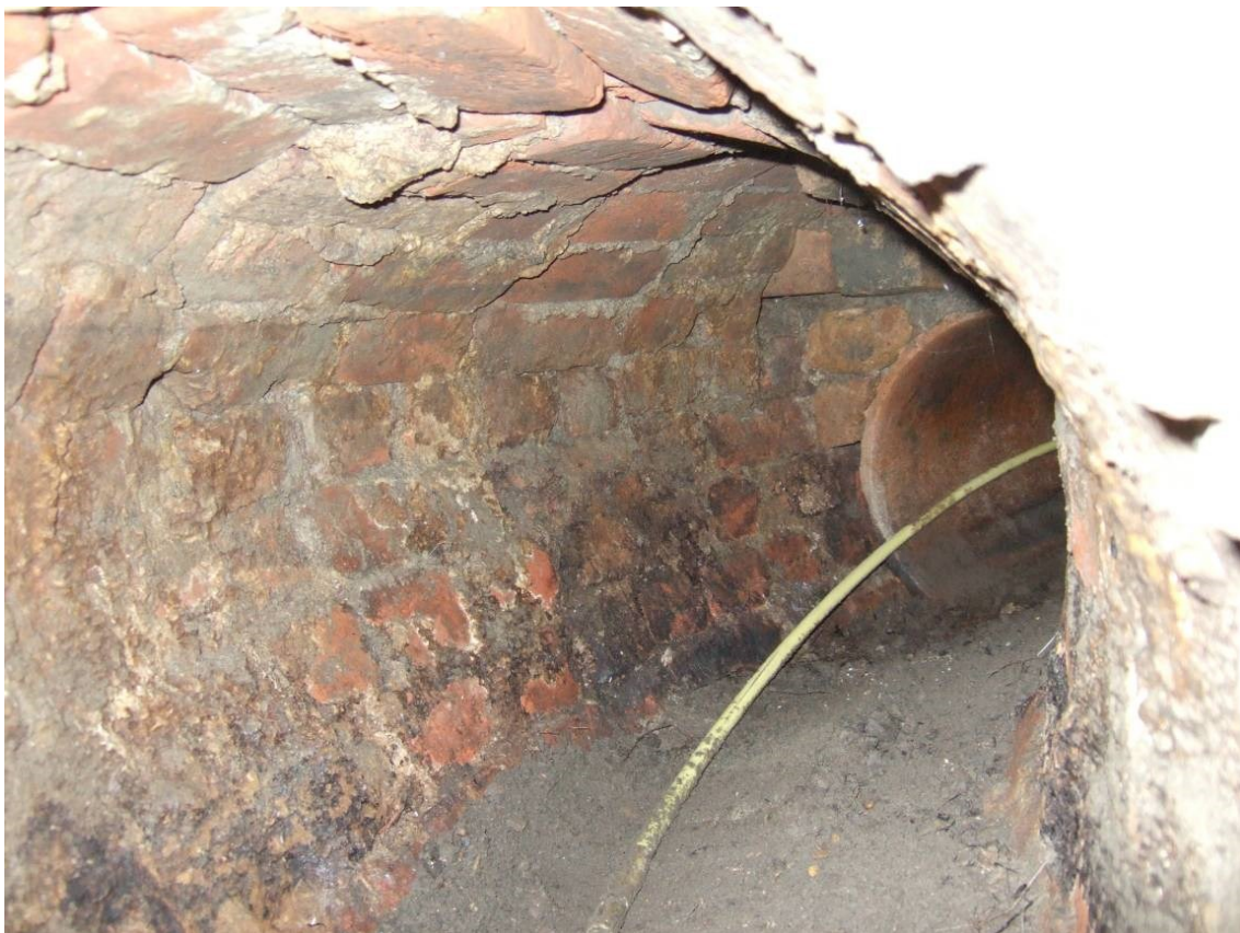
Figure 55. The inside of the culvert [C12] looking north towards Festival Walk and showing the second or northern section.
