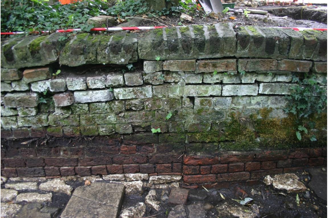
Figure 13. The bond break in the east wall of the pond.
