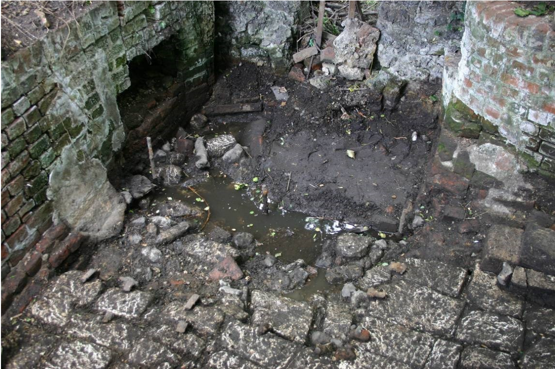
Figure 23. The floor of the rectangular pond where the stream enters. Note the damage to the floor, the iron pins used to secure the edges of the chalk blocks and, on the right, the foundation projecting from below the west pond wall.
