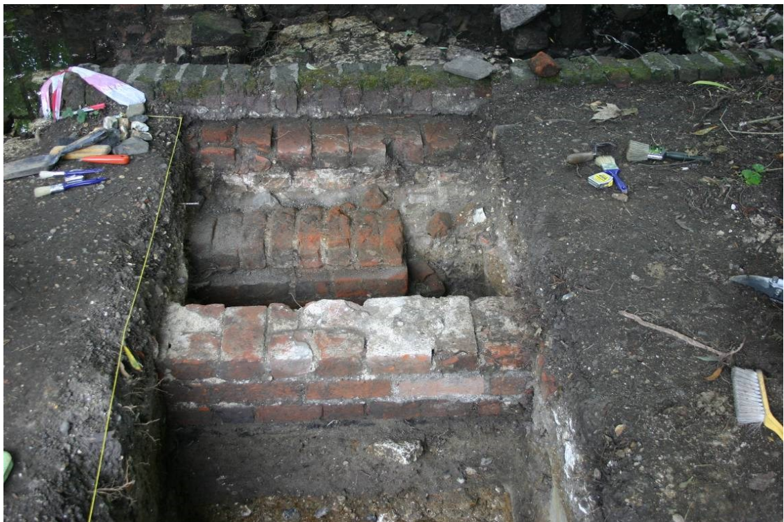
Figure 43. The three foundations exposed in trench B. From foreground to background: foundation [B5], foundation [B14] and foundation [B3] with the top of the present pond wall behind it. Looking west.
