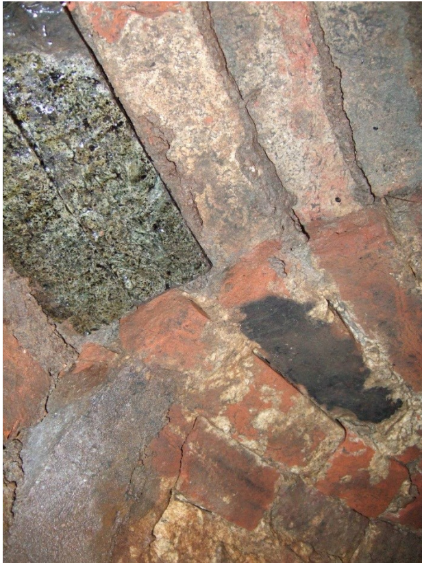
Figure 56. The junction between the two sections of culvert looking north. Note that there appears to be only one stretcher between the edge of the inspection hole at the top and the bonding break.
