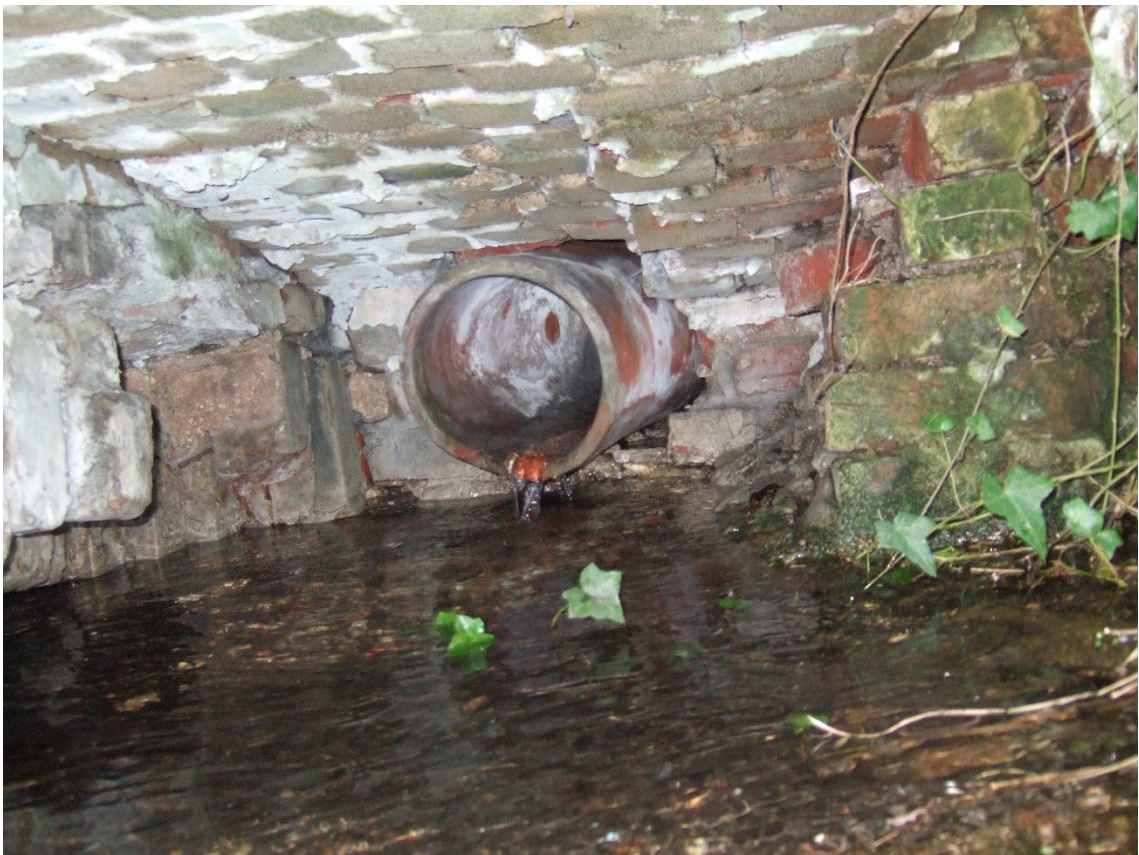
Figure 11. The south side of the entrance to the culvert under the lawn. The drain pipe runs from the oval pond shown on figure 1.
