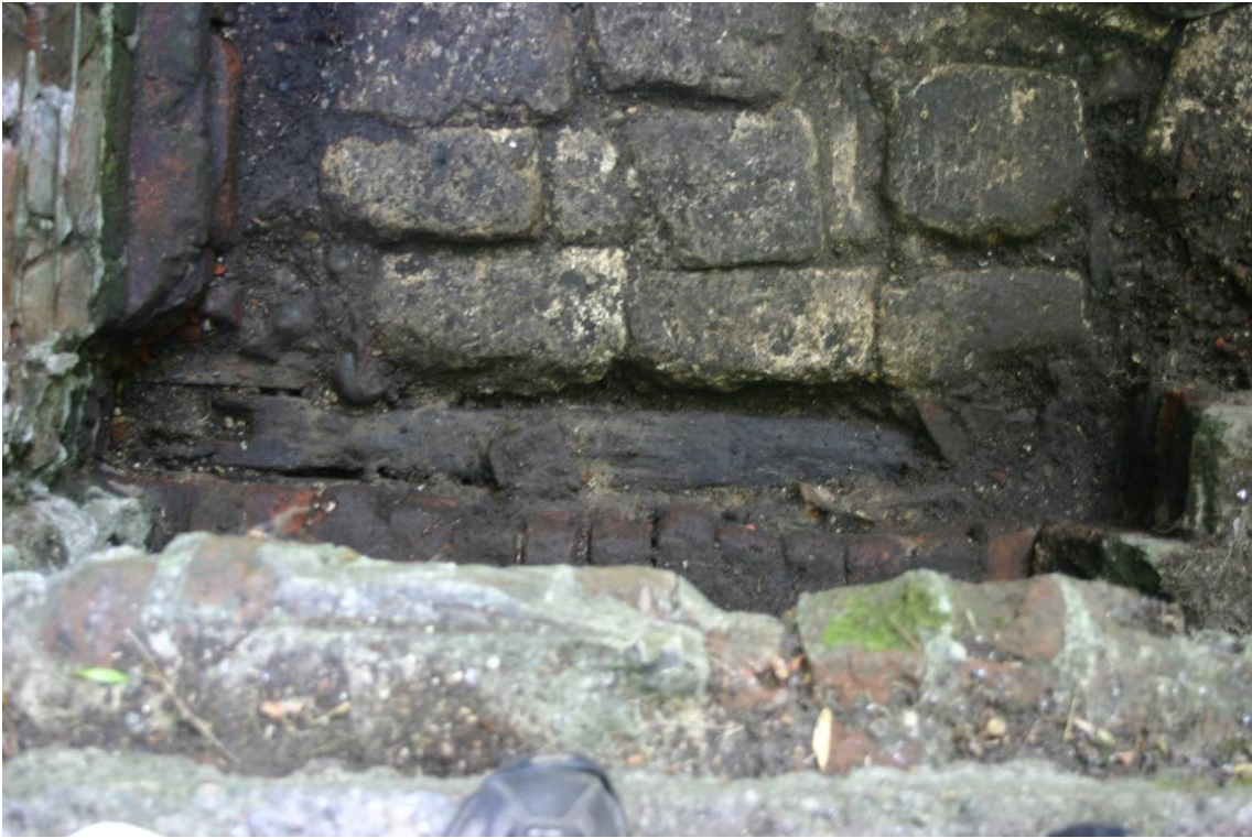
Figure 9. The remains of the sluice at the exit from the rectangular pond. Seen from above with west at the top. Note the timber sill beam and the slots for the gate.
