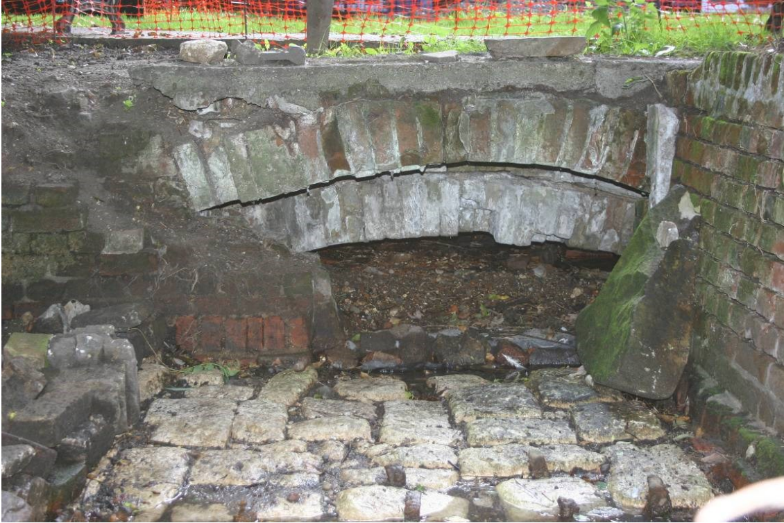
Figure 8. The exit from the rectangular pond into the culvert looking east. Note the higher outer arch and the lower inner one. The stacked brick on the far left hand side of the pond floor had been placed to retain the backfill. The Portland stone block leaning against the wall to the right has been in the pond for many years but is of unknown origin.
