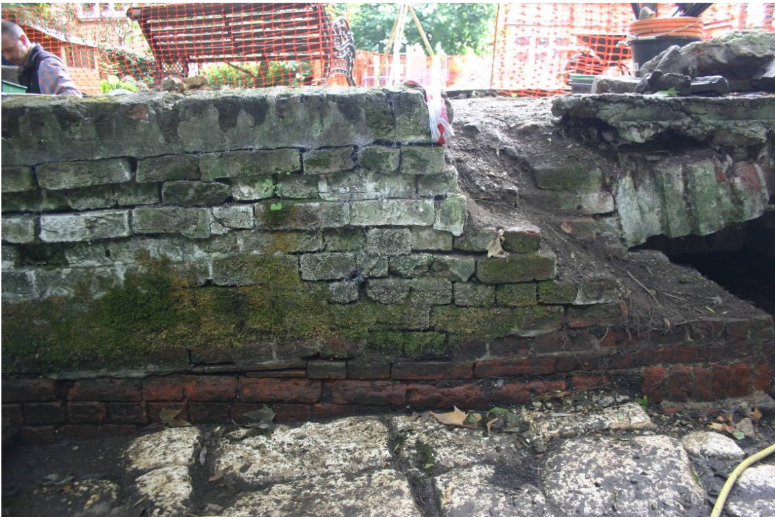
Figure 14. The south end of the east wall adjacent to the culvert. Note the packing to level up the lowest brick courses.
