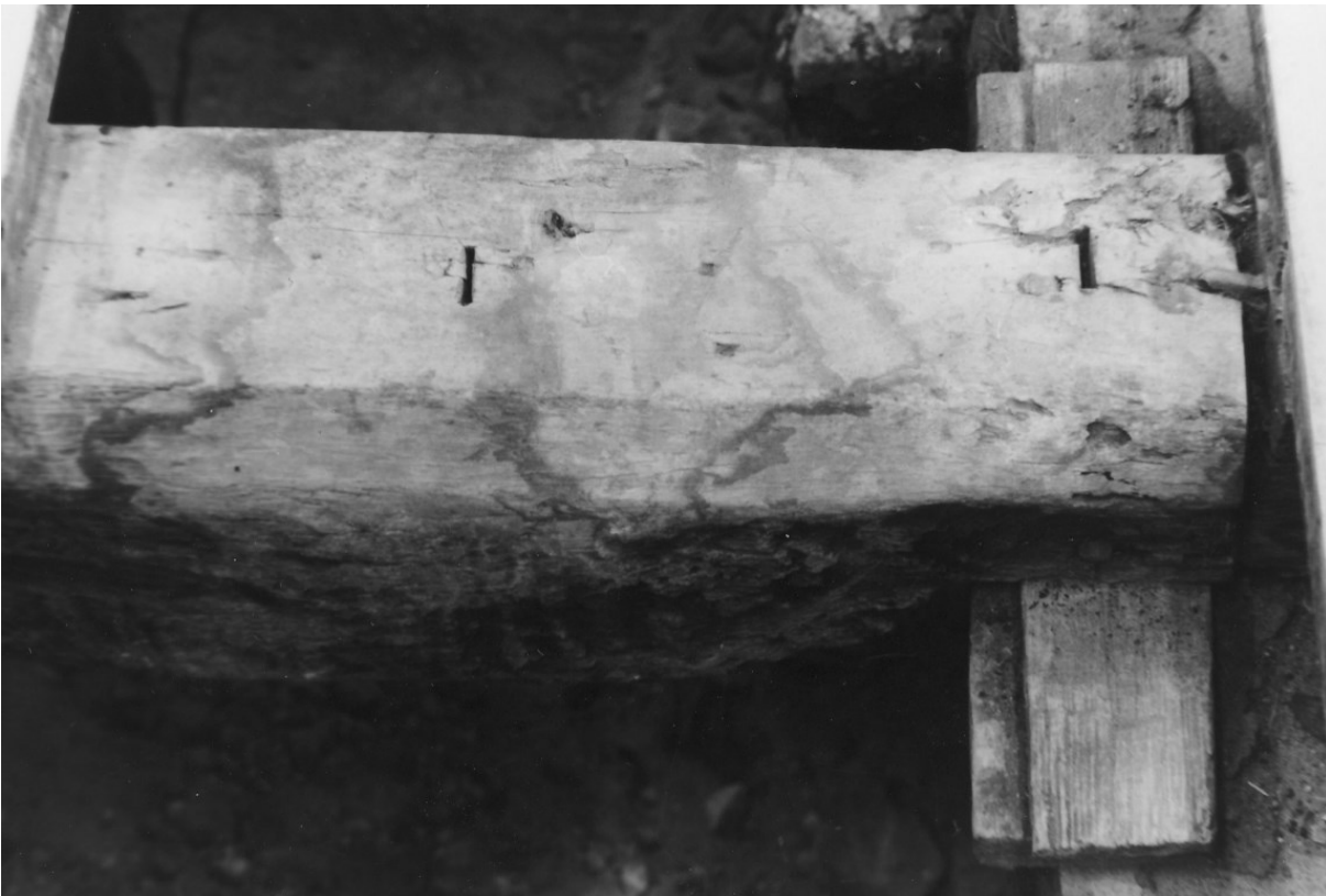
Figure 116. Upper joist 15 with lower joist 2 on the right. Looking east. Note the charring on the underside of the timber which is about 1.8m long.
