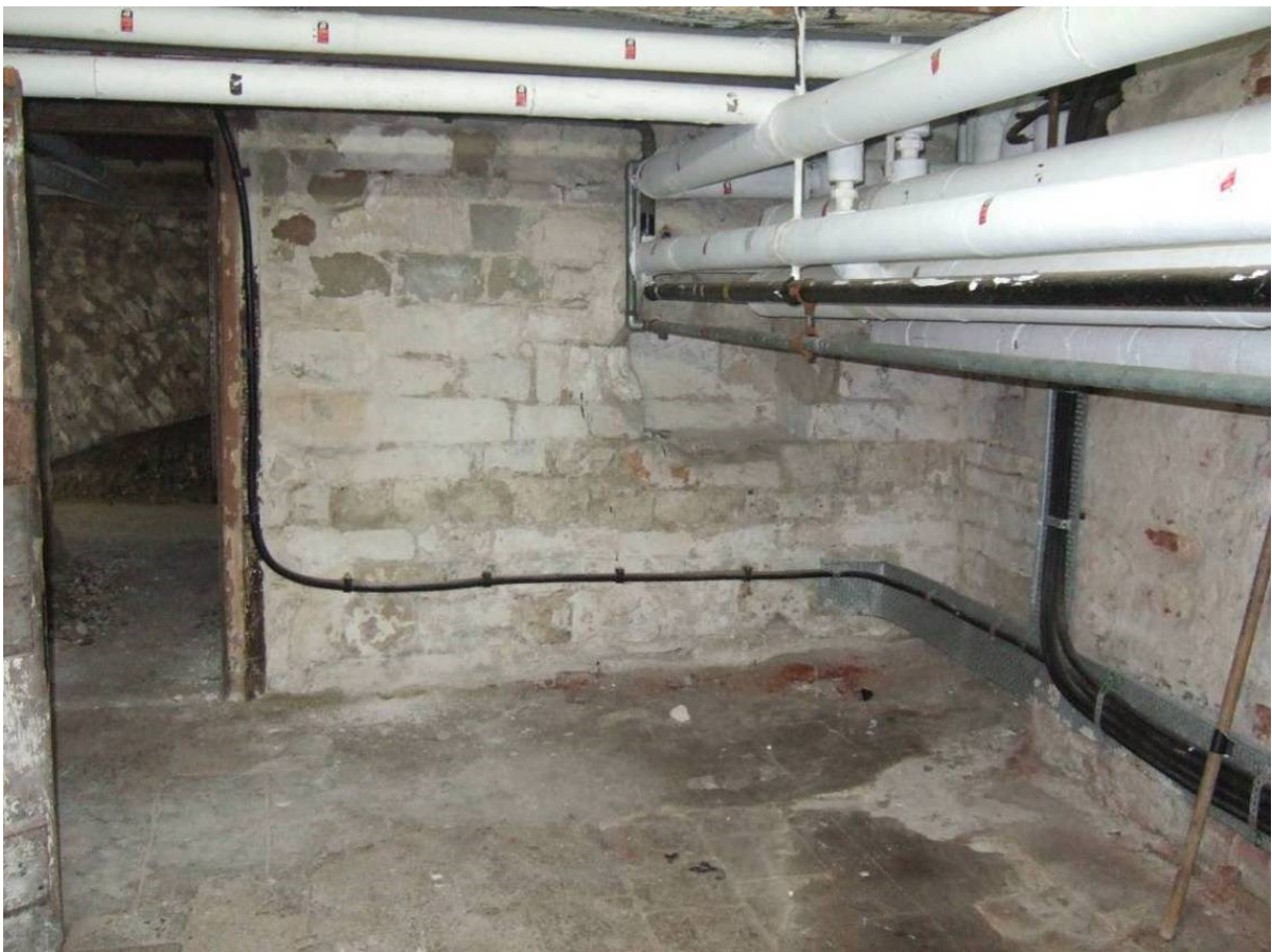
Figure 50. The south wall of cellar 6 in May 2010. The door on the left opens to the passage cut through the foundations of the former kitchen.
