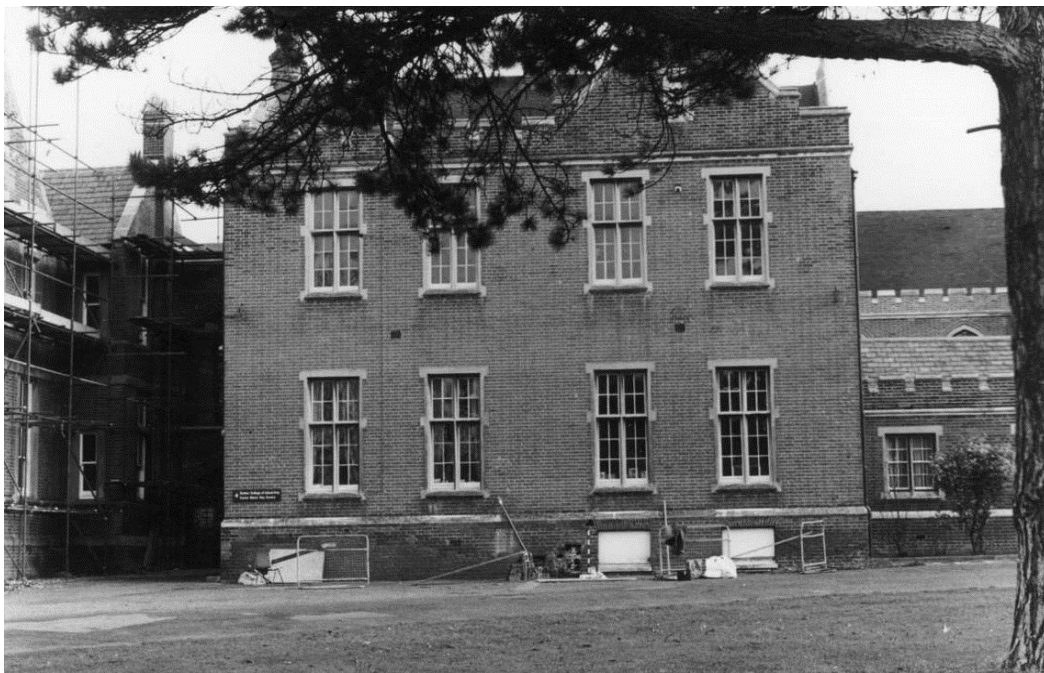
Figure 129. The west end of the north wing showing the cuts made in the repair work at the boundary between the earlier wing and the eighteenth century extension. 12 February 1984.
