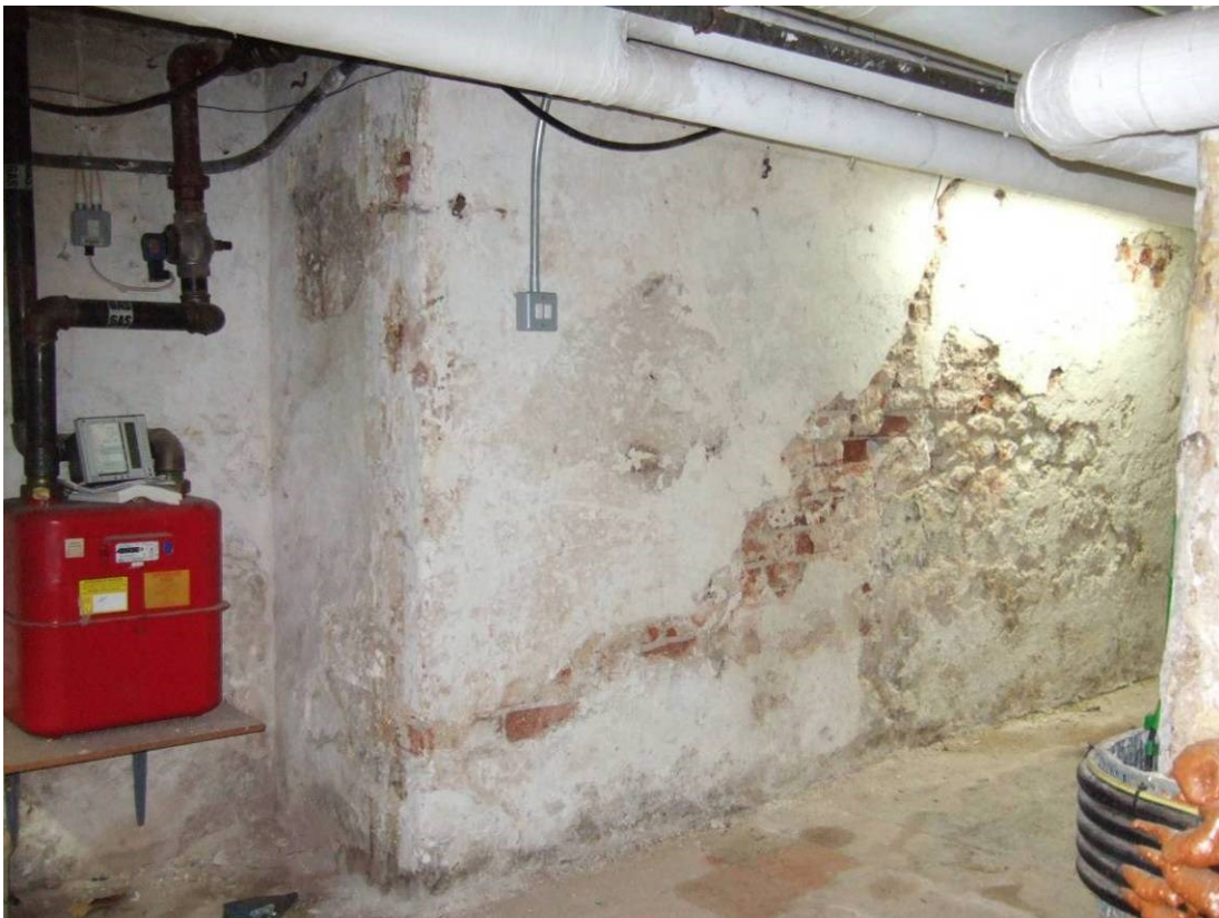
Figure 30. The east wall at the north end of the passage below the hall. Note the bond-break between the brick and the rubble.
