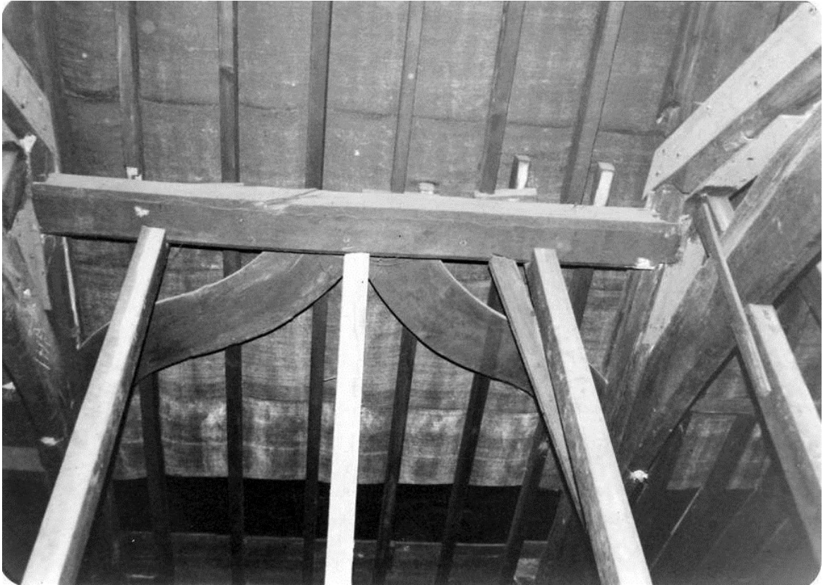
Figure 39. The surviving set of braces on the west side of the service area roof between trusses 6 and 7. February 1981.
