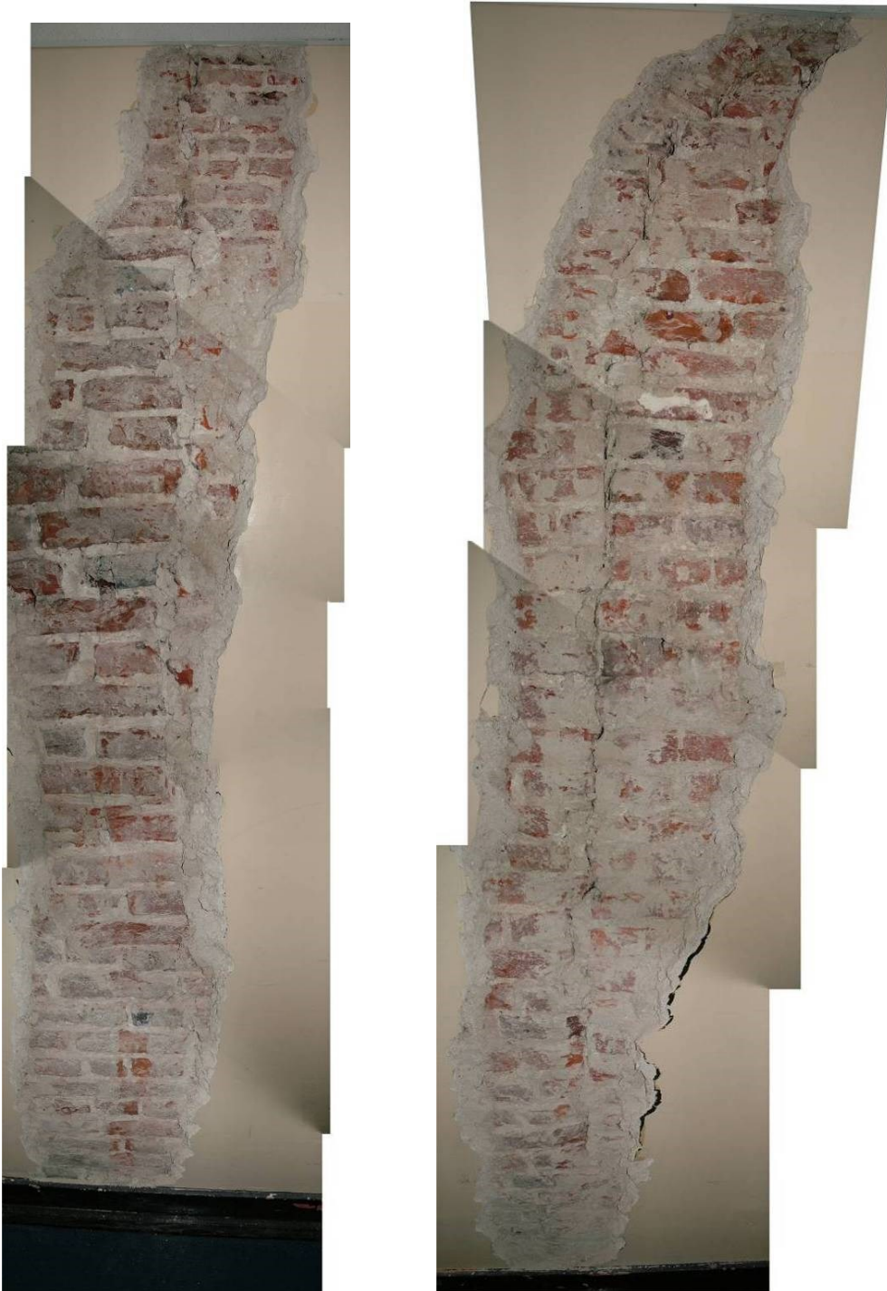
Figure 120. Photo mosaic of crack DJ (left) and crack DK (right) at first-floor level on the north side of the north wall of the hall. August 2005
