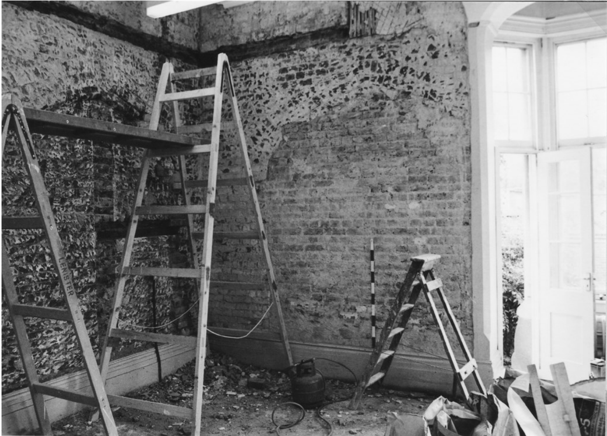
Figure 101. Part of a blocked arch in the south wall of room 134 on 1 September 1986.
