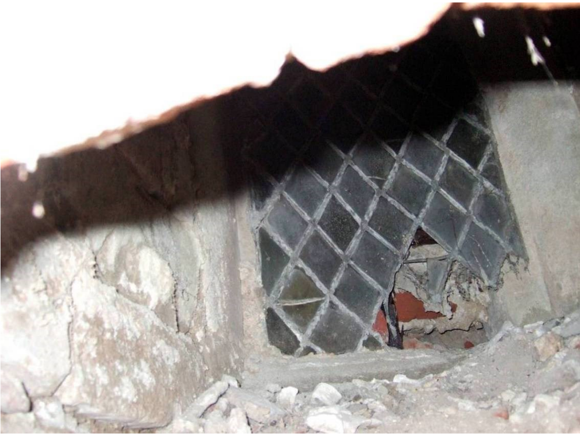
Figure 54. A bricked up window in the east wall of cellar 7 seen through a small gap between the vault and wall in September 2009.
