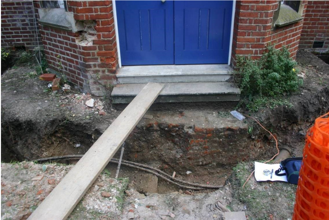
Figure 135. The trench looking west with the centre of the wing in the background. Note the brick structure below the steps.
