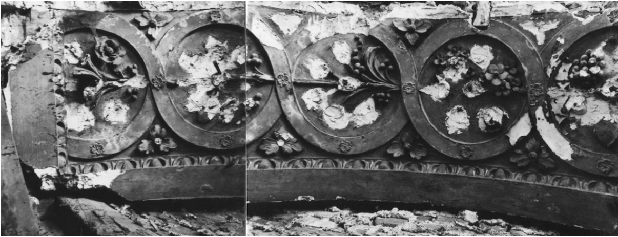
Figure 35. The underside of the opening which formerly connected the northeast corner of the hall to the parlour.
