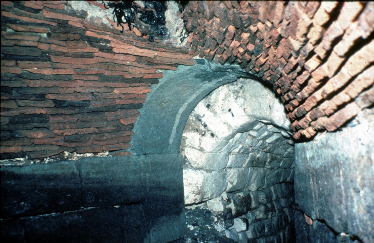
Figure 77. The chamber at the end of F1 showing the vault and the exit towards the main culvert.
