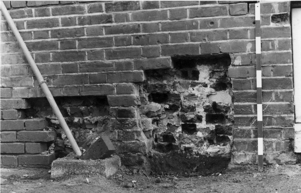
Figure 130. The west end of the north wing showing the cuts made in the repair work at the boundary between the earlier wing and the eighteenth century extension. 12 February 1984.
