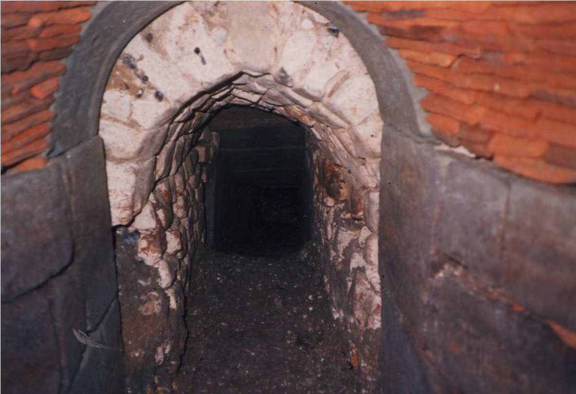
Figure 76. Culvert side drain F1 looking from the end chamber south towards the main moat culvert.
