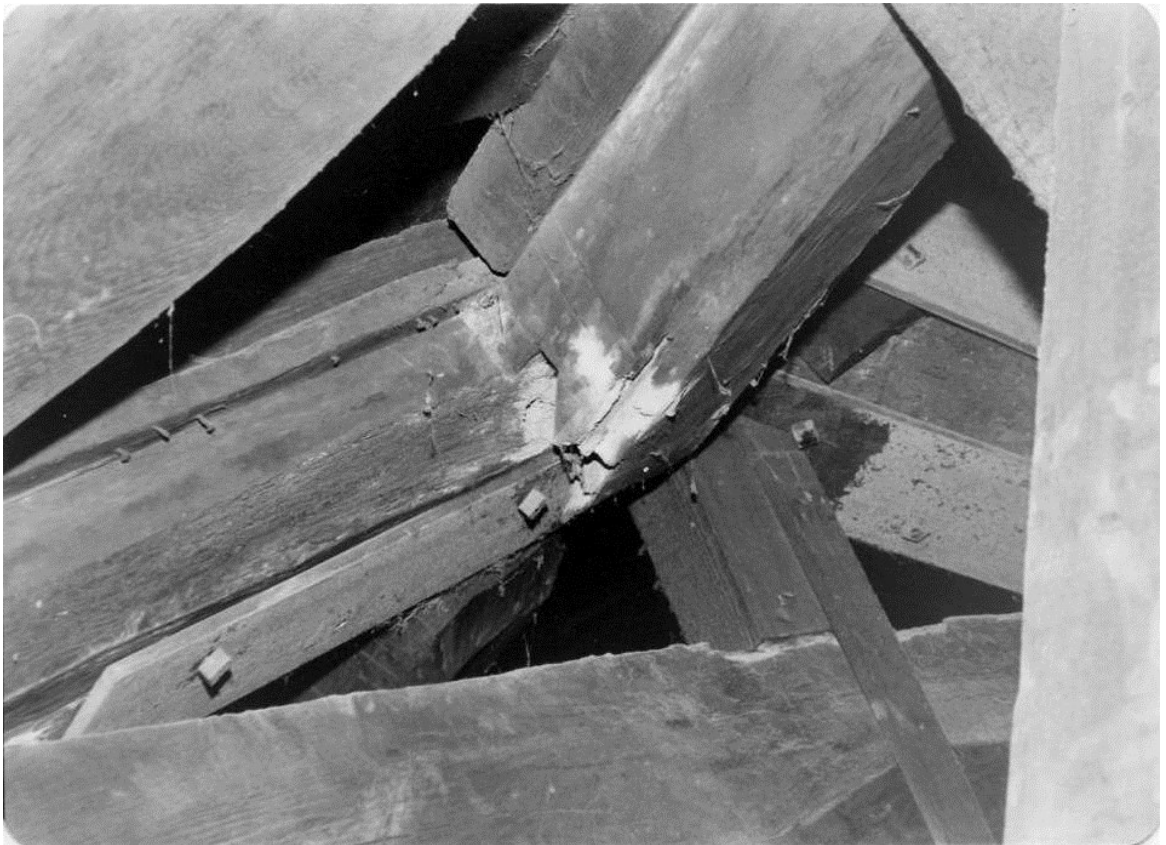
Figure 40. The west side of the service area roof showing the junction between the purlin and the south side of truss 6. February 1981.
