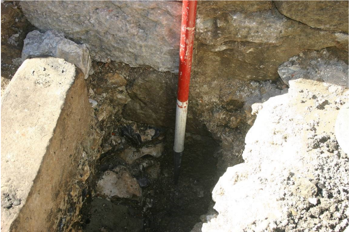
Figure 100. The junction between the moat wall [CEZ24] on the left and abutment [CEZ23] in the background.
