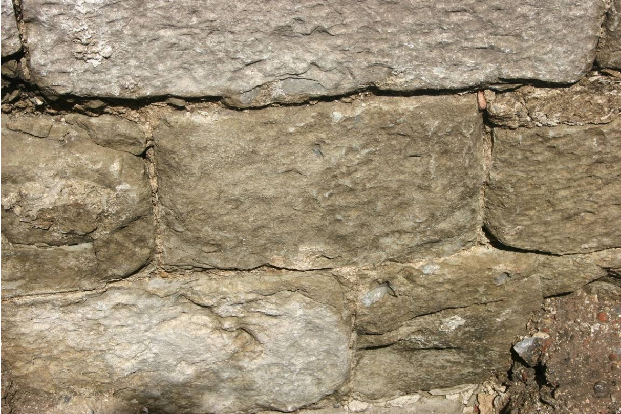
Figure 94. The stone blocks on the side of the abutment in trench CEZ.
