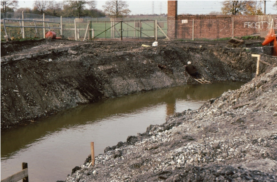
Figure 35. The two culverts (one behind Ron Green – the kneeling figure) and the section cut for the re-aligned river channel.
