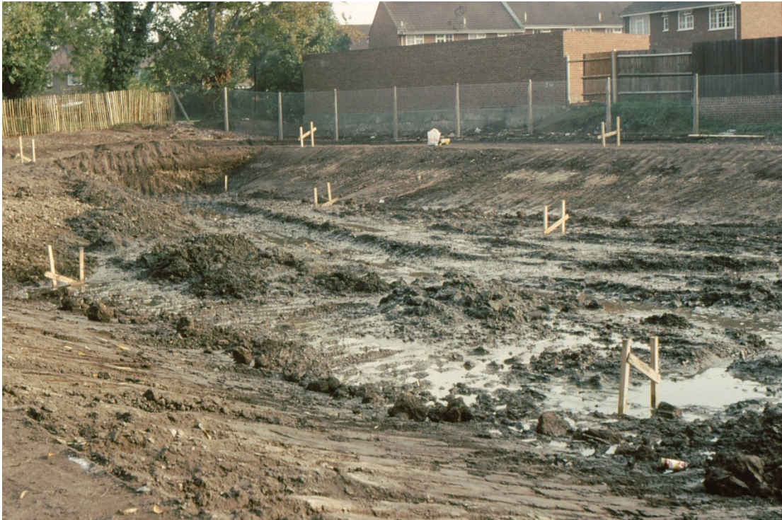
Figure 27. The excavation of the new pond with the section FC in the background. Looking southeast.
