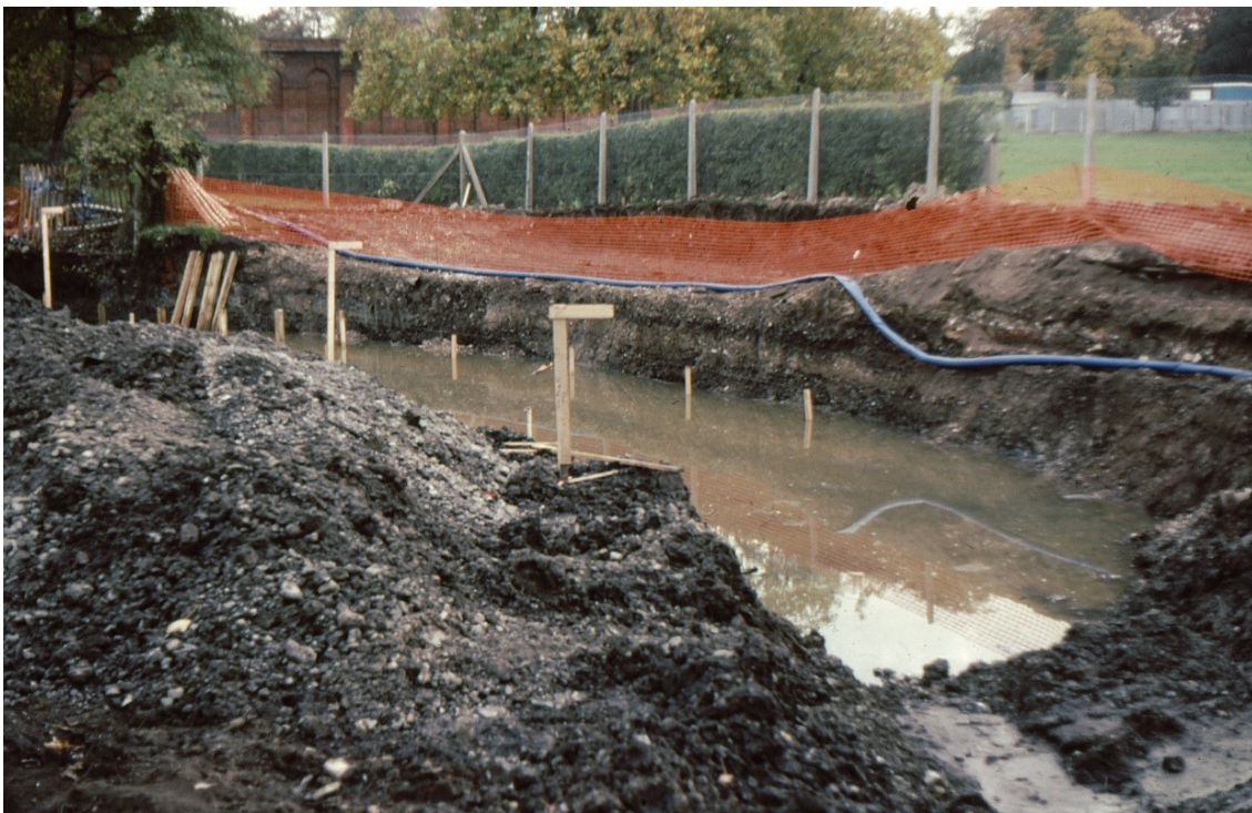
Figure 32. The realigned channel where the river turns north. The view looks south and somewhat west with the Orangery wall in the background.
