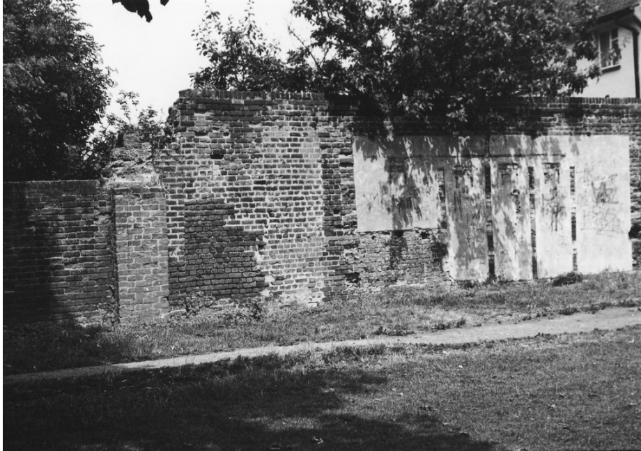
Figure 10. The west end of the north wall showing the remains of a pillar of uncertain date and the scars from the demolished swimming pool changing cubicles.
