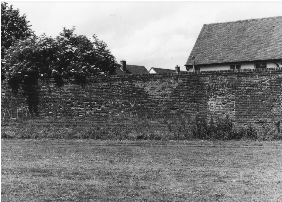
Figure 11. The north wall of the eastern end of the central garden in 1986 showing the blocked door.
