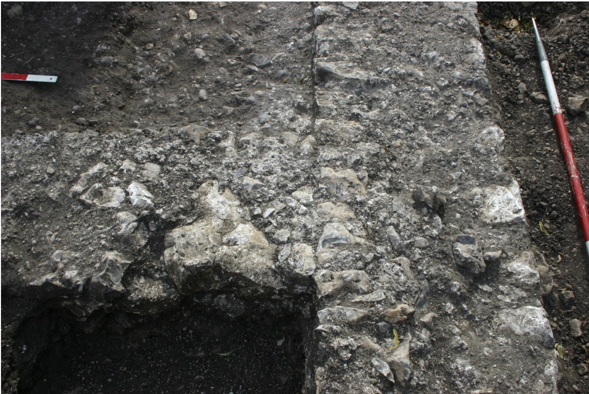
Figure 19. Trench A: the junction between the main wall of foundation [5] (right) and projection P4 (left).
