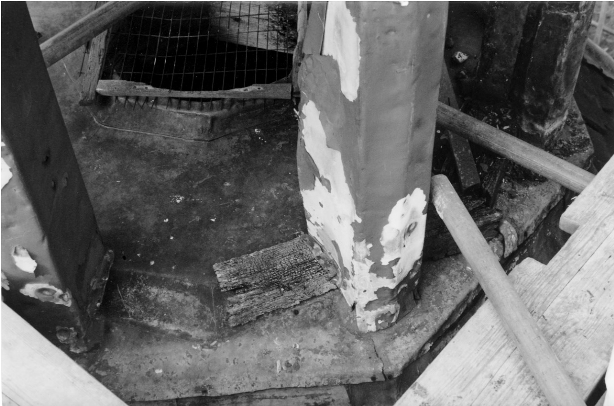
Figure 14. The base of the turret. The inner half of the column rested on a timber ring beam which in turn rested on lead capping at the top of the main roof.
