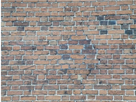
Figure 45. The scar on the west wall where the first-floor bridging beam was inserted.
