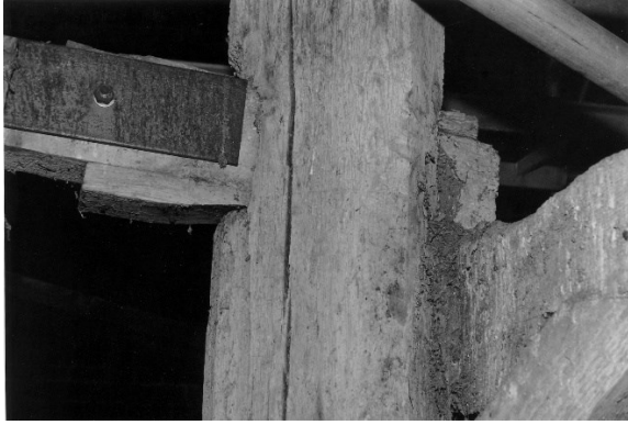
Figure 48. The joint between the potence post and the horizontal timber which supports the upper end of the ladder.
