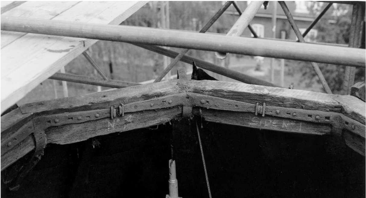
Figure 21. The ring beam at the apex of the roof showing the iron ties binding the structure together.
