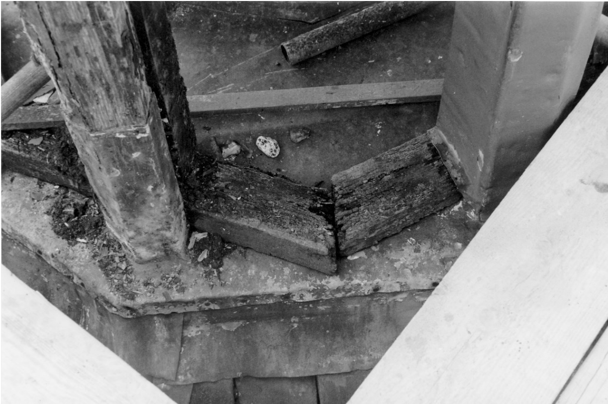
Figure 15. A further view of the base of the turret showing the inner and outer timbers of the column on the left. The inner one rested on the ring beam.
