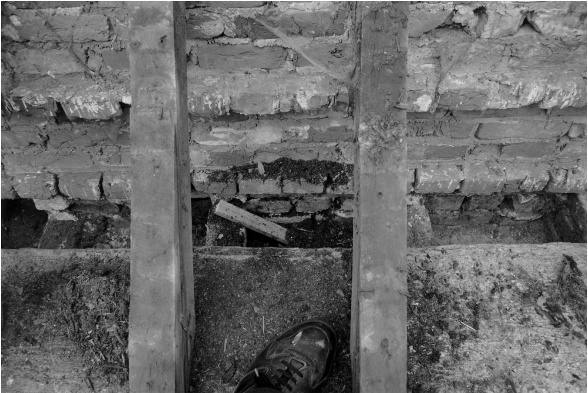
Figure 44. The top of the nesting boxes. The wall plate is at the bottom of the photos and the nesting box wall at the top.
