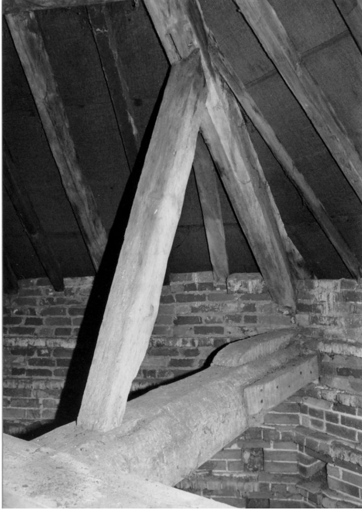
Figure 20. The east end of the main tie-beam at corner 2 showing the brace between it and the principal rafter. Note that the mortise on the underside of the rafter is for a wider brace. This was the brace which was in place before the 1997 repairs.
