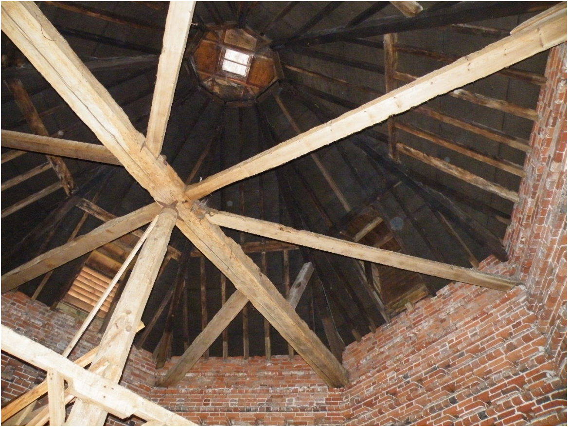
Figure 16. The roof frame. The western end of the main tie-beam can be seen bottom centre.
