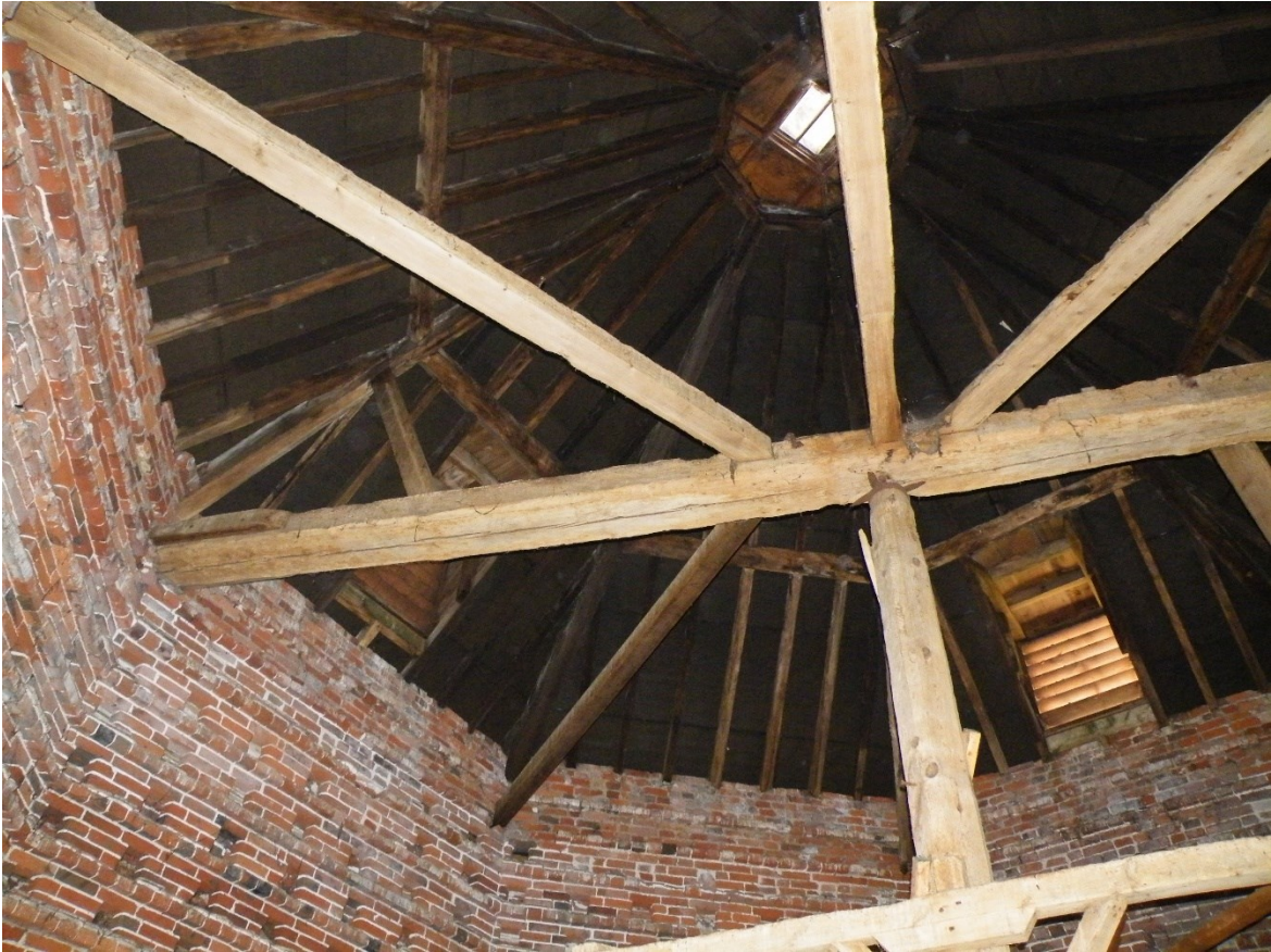
Figure 19. The east side of the roof with the east end of the main tie-beam centre left.
