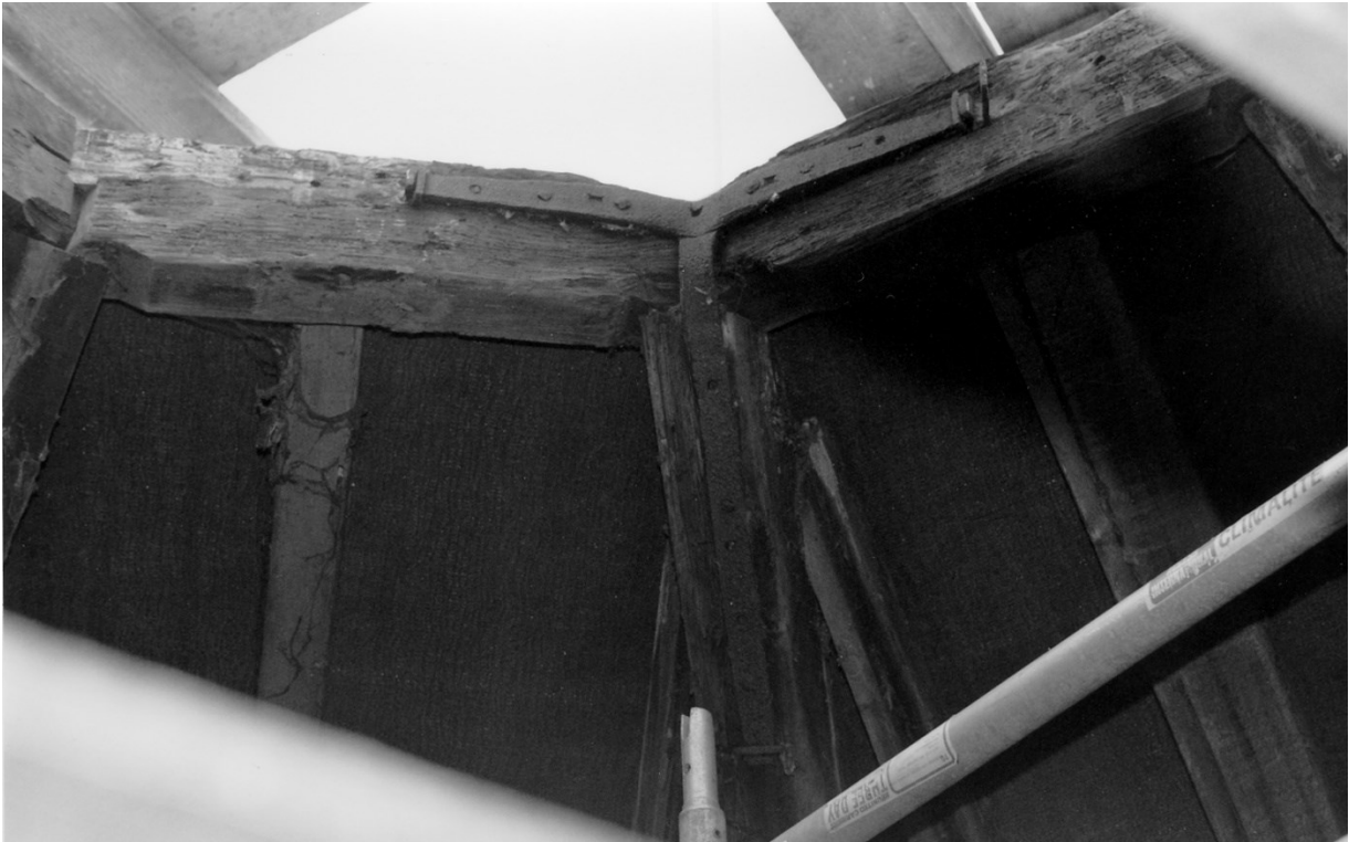
Figure 23. The underside of the roof apex showing the ring beam and the iron ties joining it together and linking it to the top of the principal rafters.
