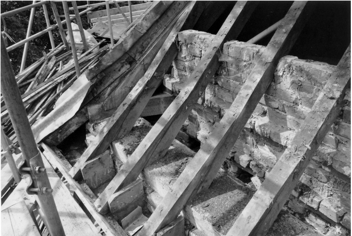
Figure 42. The top of the wall showing the common rafters and the sprockets which support the roof above the eaves and end against the board forming the top of the cornice. The common rafters end on the wall plate which rests on the brick outer wall. The inner wall which forms the front of the nesting boxes rises up to meet the underside of the rafters.
