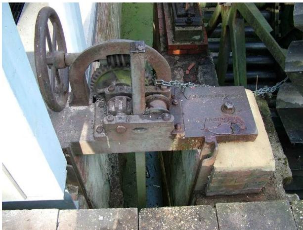
The spillway gate between the two wheel-pits must have been replaced at the same time as it has Armfield's name on it.
