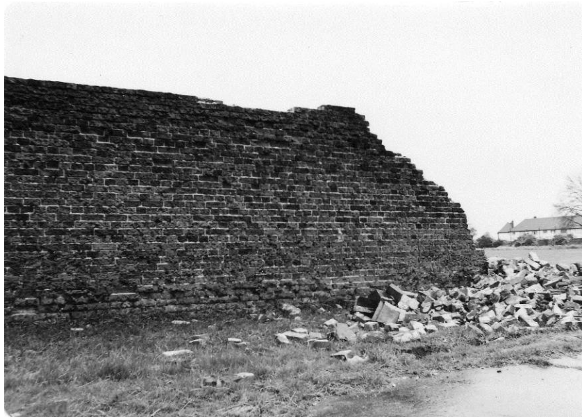
Figure 64. The remains of the wall between the north gate and river on 3 May 1981. Note the bond break adjacent to the gate pier. The wall has now been replaced by a hedge.
