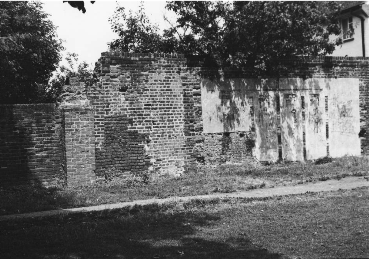
Figure 68. The west end of the north wall in 1986 showing the remains of a pillar of uncertain date and the scars from the demolished swimming pool changing cubicles.
