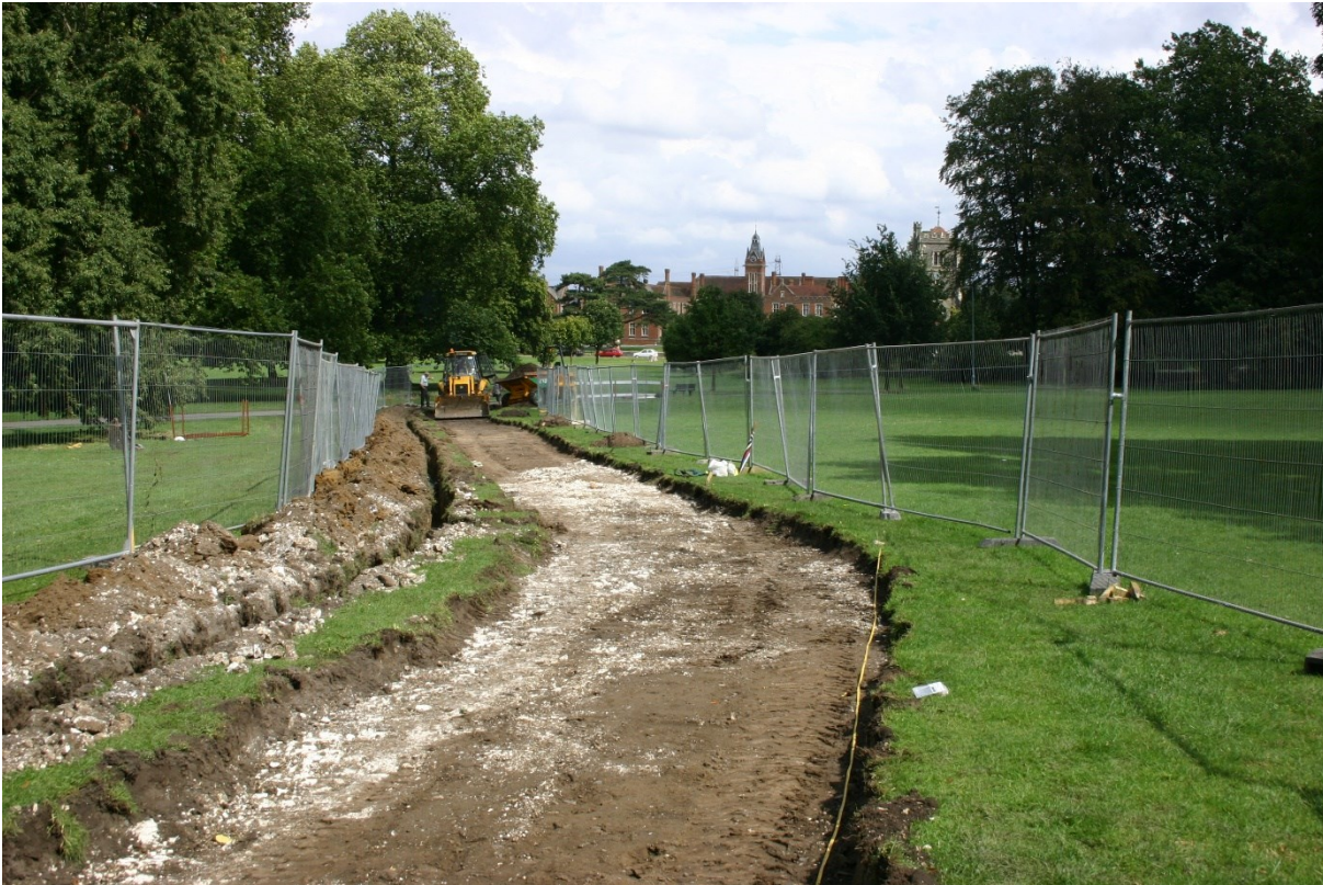
Figure 42. The chalk foundation exposed during the construction of the cycle track in 2004.
