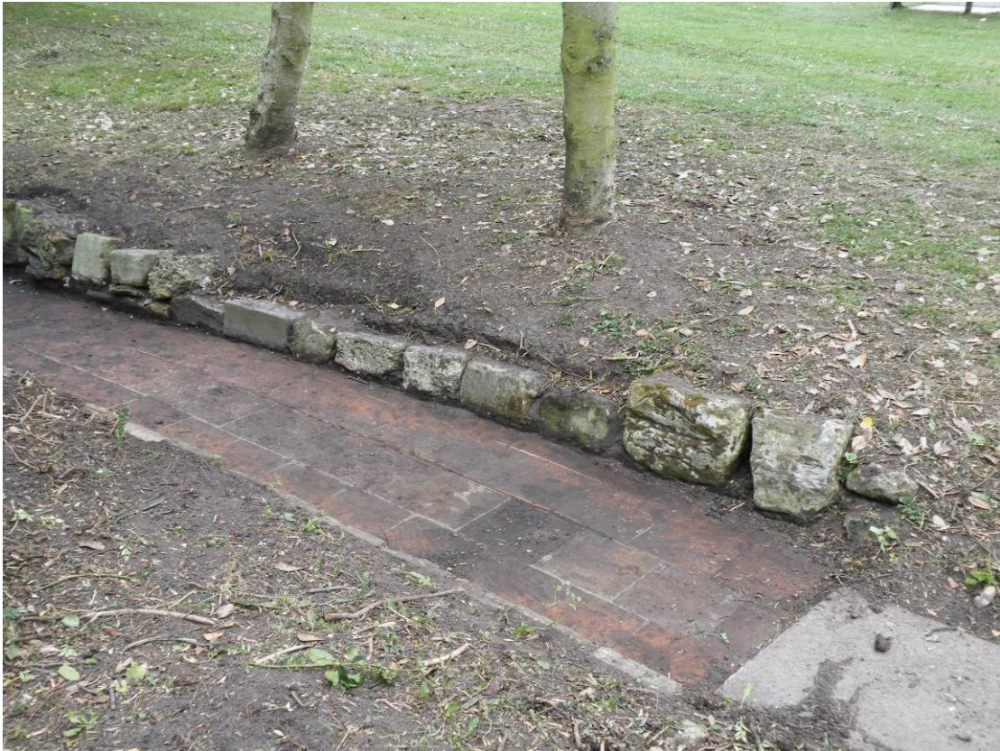
Figure 121. The western end of the fernery in 2015 showing the south wall overlying the floor tiles.
