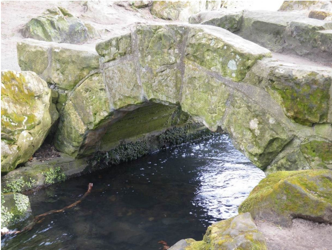
Figure 133. The bridge over the spillway in the rockery in 2013. Note the concrete arch.
