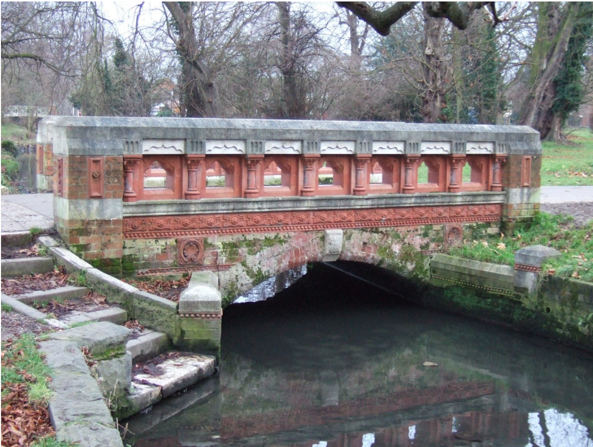
Figure 27. The downstream side of Canon Bridges' Bridge in 2006. Much of the terracotta is restoration following damage in the 1987 gale.
