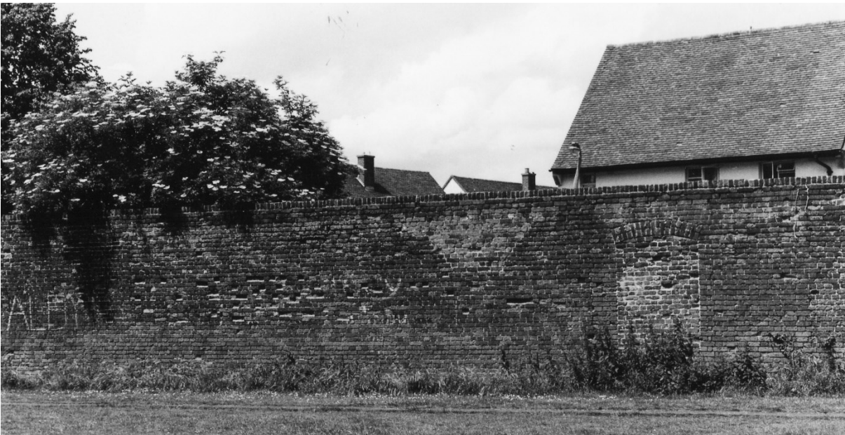
Figure 69. The north wall of the eastern end of the central garden in 1986 showing the blocked door.
