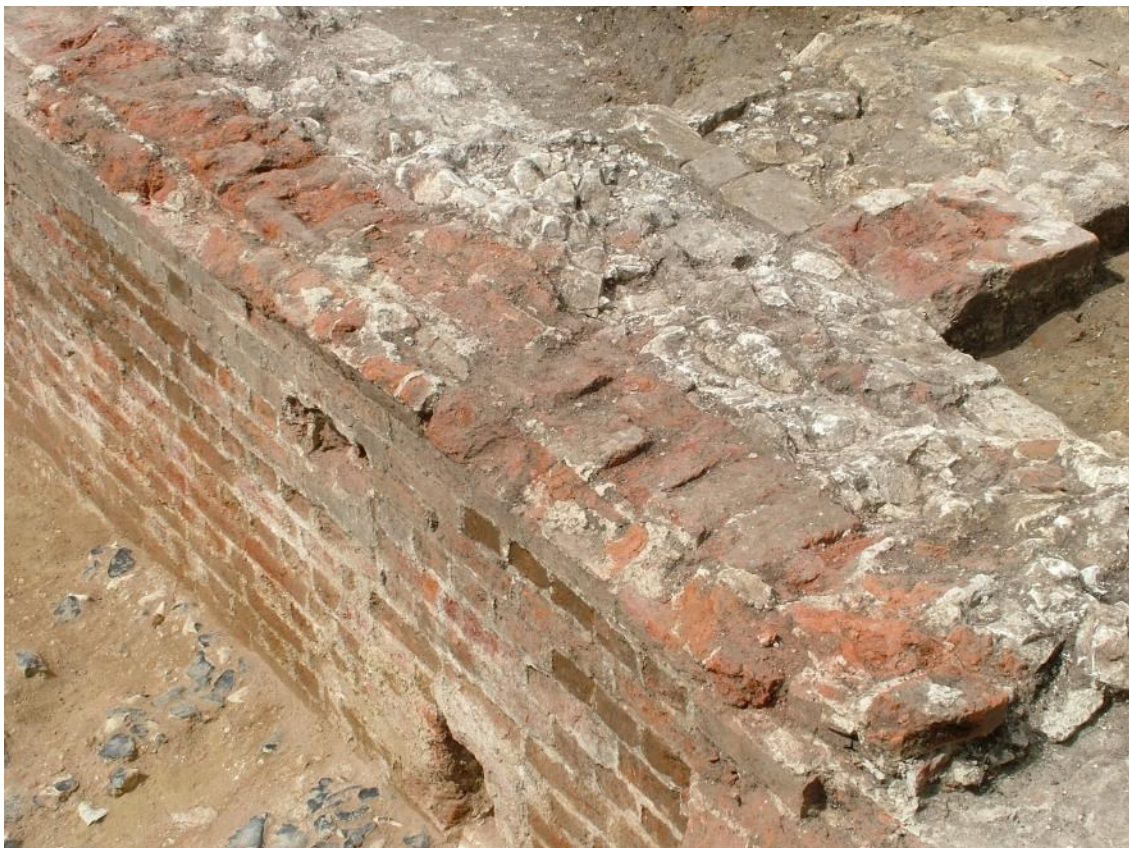
Figure 4. The north wall of cellar 1 with a line of inward sloping bricks which suggest that the cellars had originally been vaulted.
