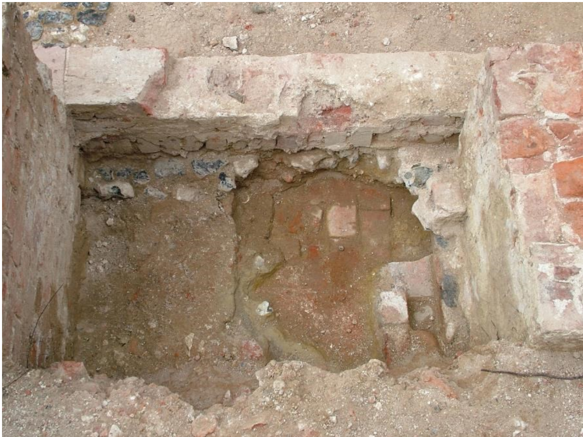
Figure 18. The door between cellars 1 and 5. The floor is of flint set in sand with brickwork below.
