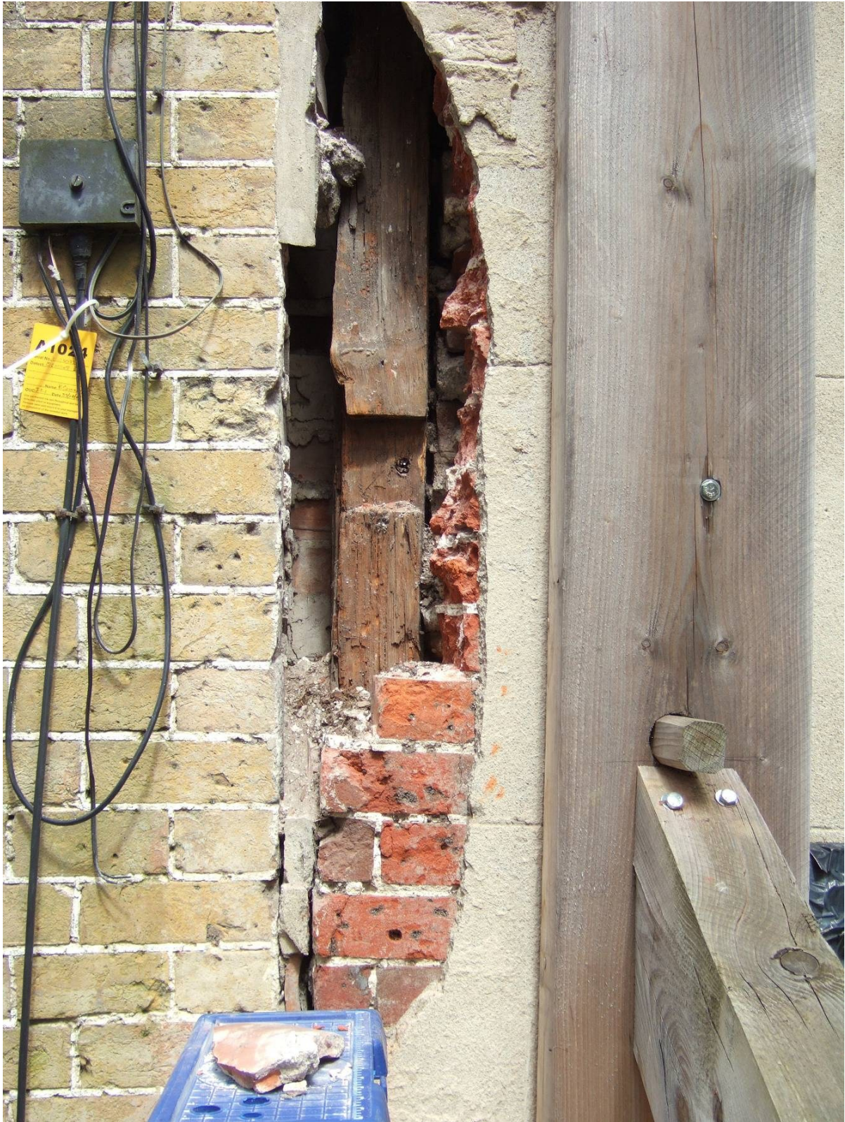
Figure 14. Detail of the western end of the south wall of the south wing showing the timber post with the halving and the brickwork behind it.
